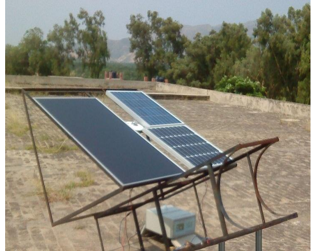
Figure 1- Orientation of PV Modules
