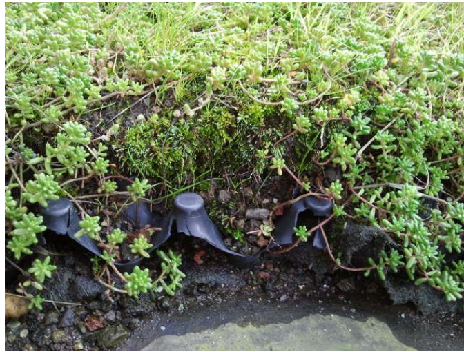
Figure 2: A green roof with different layers at Delft University of Technology, Delft, the Netherlands.
