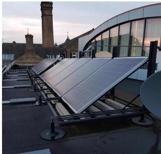
Fig. 1. Examined PV system installed at the University of Huddersfield, United Kingdom
