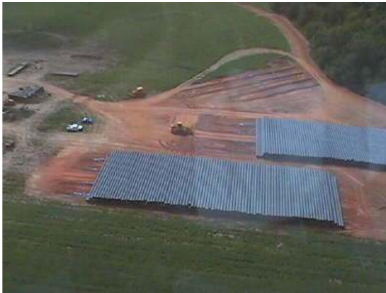
FIGURE 3.3-5 Pipe Segments in a Material Laydown Area (Source: Photo courtesy of U.S. Pipeline, Inc. Reproduced with permission.)
