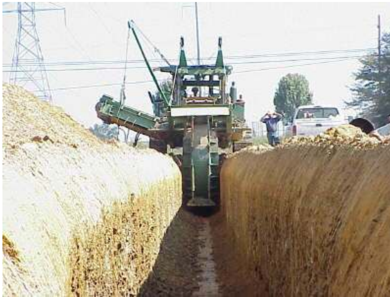
FIGURE 3.3-9 Pipeline Ditching (Source: Photo courtesy of U.S. Pipeline, Inc. Reproduced with permission.)
