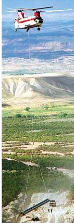
FIGURE 3.3-8 Delivering Pipe Segments to the Construction Site in Rugged Terrain May Require Special Equipment (Source: Photo courtesy of U.S. Pipeline, Inc. Reproduced with permission.)
