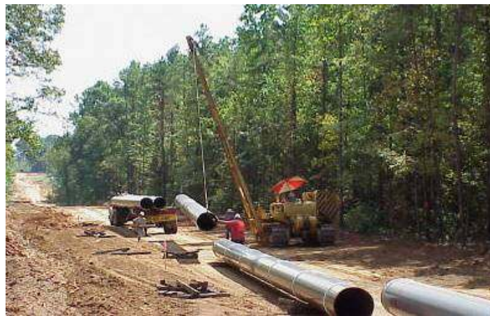
FIGURE 3.3-7 Stringing Pipe along the ROW (Source: Photo courtesy of U.S. Pipeline, Inc. Reproduced with permission.)
