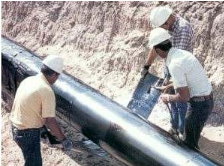
FIGURE 2.1-1 Coating Newly Installed Pipe for Corrosion Control (Source: Photo courtesy of Corrosion Control Products Co. Reproduced with permission.)
