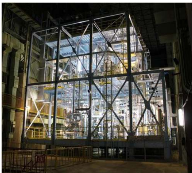
Figure 15. Night view of the ELTL under operation until October 2014 in the JAEA premises of Oarai.
