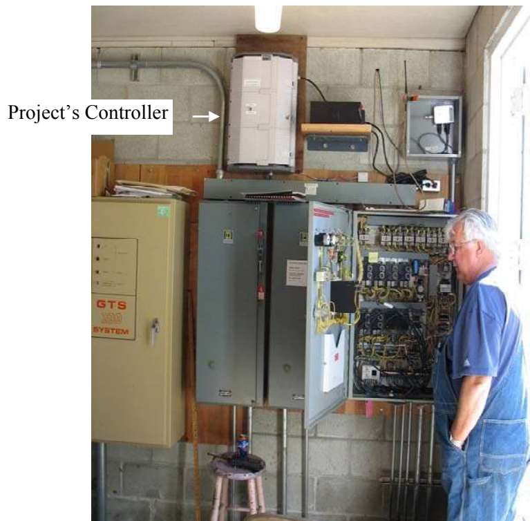
Figure 5.4. Control Panels at the Sekiu Pumping Station
