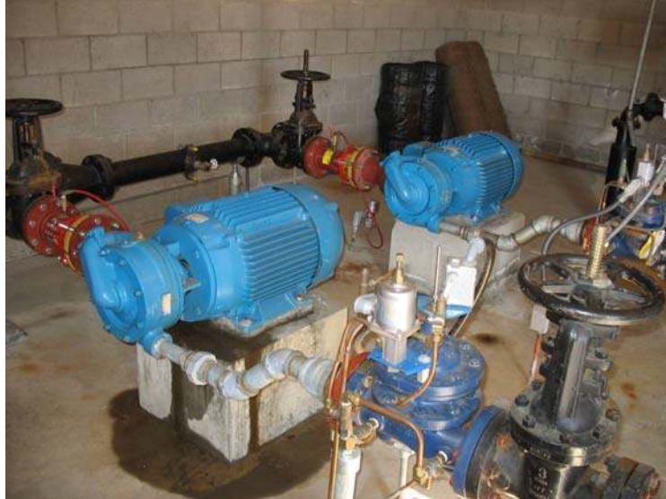
Figure 5.1. Pumps at the Sekiu Water Pumping Station
