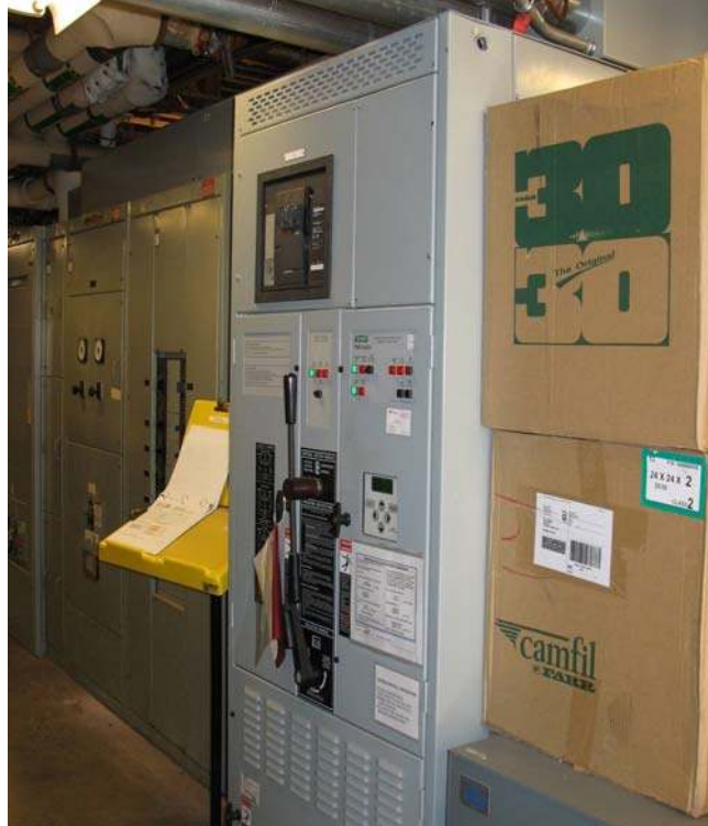
Figure 6.3. Upper Generator Power Transfer Switch at PNNL's MSL
