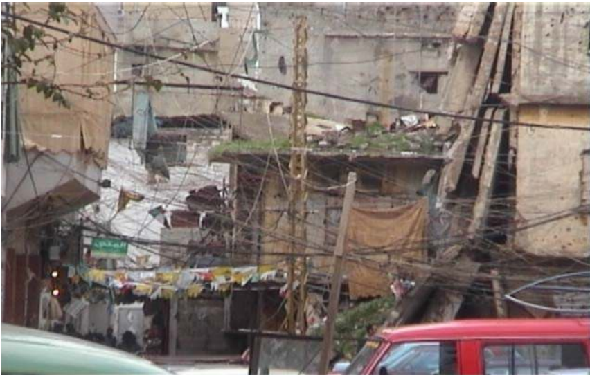
Figure 18: Shatila Camp/Beirut: A Web of electricity cables and wires cover the narrow streets of the overpopulated refugee camp
