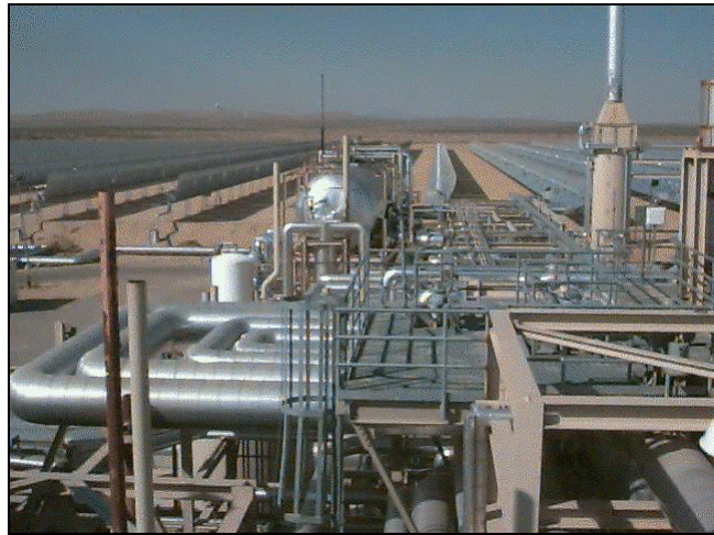
Figure 11. SEGS VI power block
