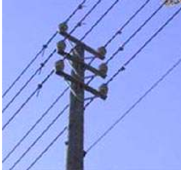
Fig. 2.4 Double 20 kV PAS line – no wider than a normal single bare copper line
