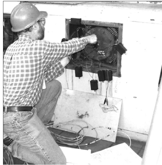
Figure 13 – RTD's Connections for Partial Discharge Detection – On Line
