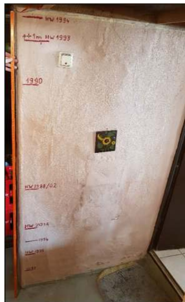
Fig. 12 Flood markings in the cellar of a study participant in the flood area in Eberbach, Germany. In 1993, the water filled the whole cellar and reached the first floor. The residents have painted their cellar with special oil paint and only store belongings in the cellar that can be removed easily. Photograph by C. Klonner, Eberbach, July 2018
