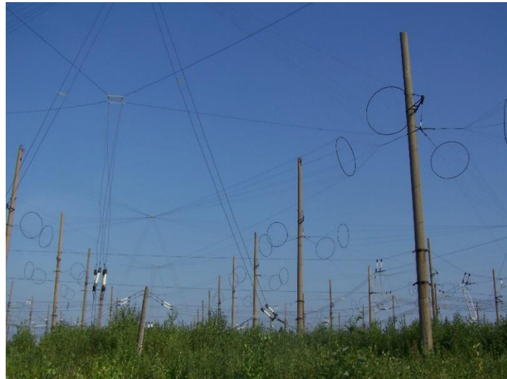
Figure 2.2. A view of the SURA antenna array.
