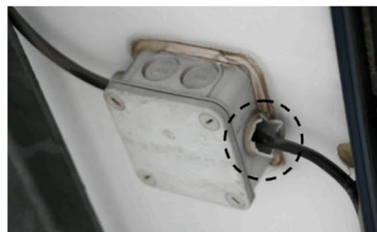
Figure 2. Cracks in the terminal boxes appeared during the first 13 years of operation.
