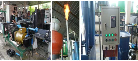
Figure 7. Checking quality of producer gas and running generator.
