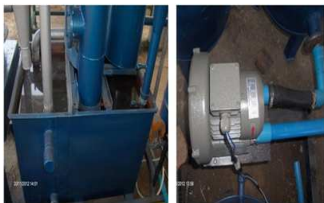
Figure 4. Heat exchanger and producer gas transmitter system.
