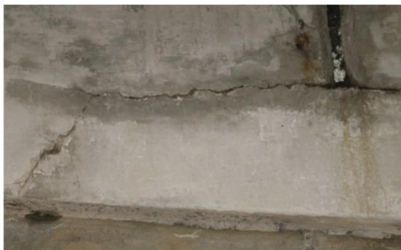
Figure 4: Superstructure cracking (BAST, 2015)
