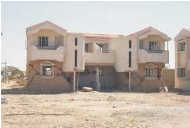
Fig. 26. Row of semi-detached houses in Samkhiali; note the open spaces in the first storey, the masonry infill wall at the back, and the slender columns supporting the front of the building.
