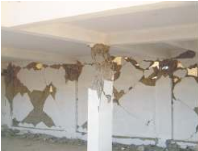
Fig. 23. The hinge regions of the columns in the open first storey of this building in Anjar are heavily damaged; complete collapse of the building was prevented by the presence of a few infill walls, which although heavily damaged remained in their place.
