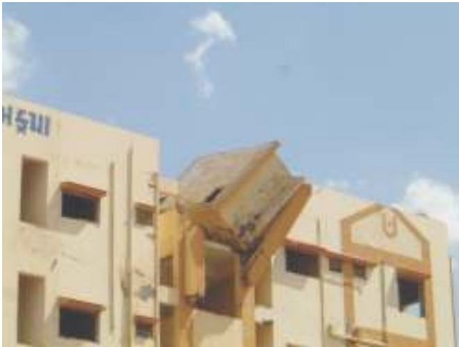
Fig. 30. A water tank supported by four short columns projecting above the roof collapsed during the earthquake.
