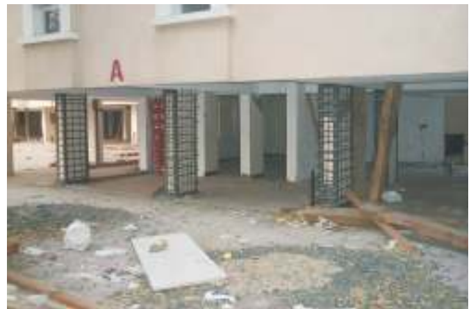
Fig. 14. Repairs to damaged columns in the first storey of the Shikhara building.
