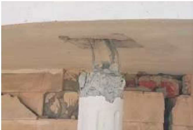
Fig. 27. Details of the column supporting the front of the building shown in Fig. 26.
