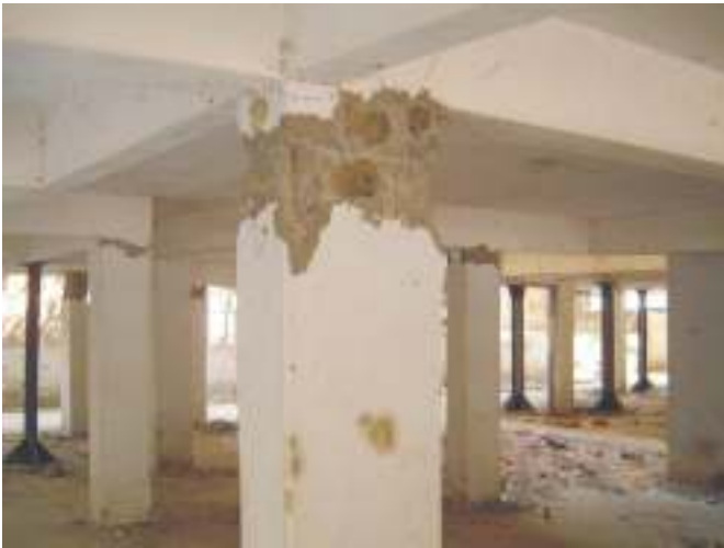
Fig. 11. Damage suffered by the open first storey columns in concrete frame building.
