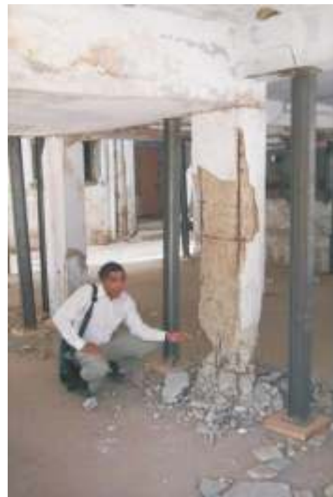
Fig. 21. The damaged first storey of the building on the right-hand side of Fig. 20.
