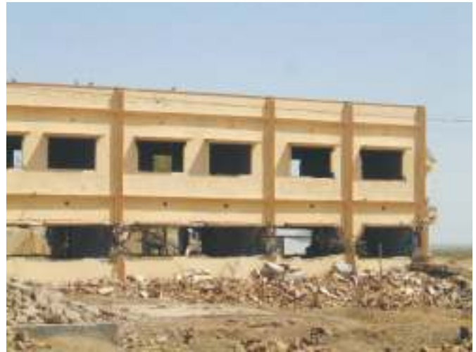
Fig. 24. Failure of reinforced concrete short columns in a school in Bhachau.
