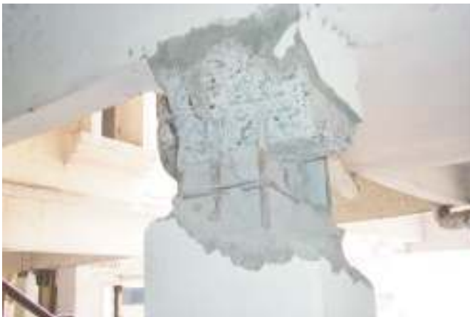
Fig. 12. The hinge in a first storey column showing the steel reinforcement.
