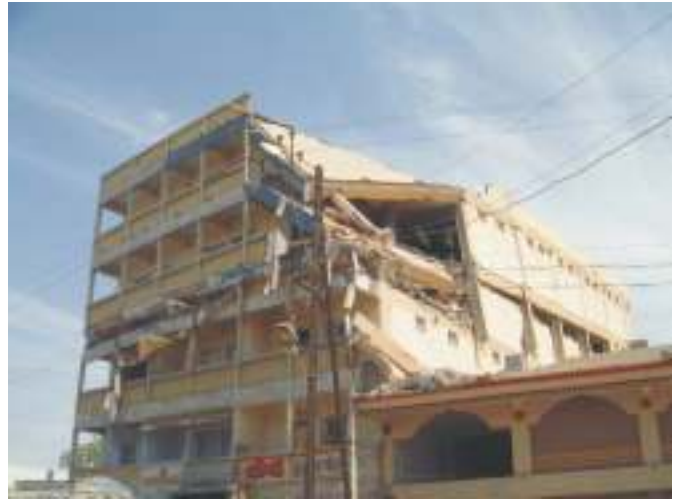
Fig. 28. The fourth storey of this six-storey building in Bhuj collapsed bringing the topmost two storeys down and causing more extensive damage to one corner of the building.
