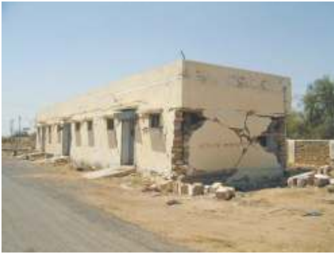
Fig. 9. Damaged control room building at the Samkhiali substation.
