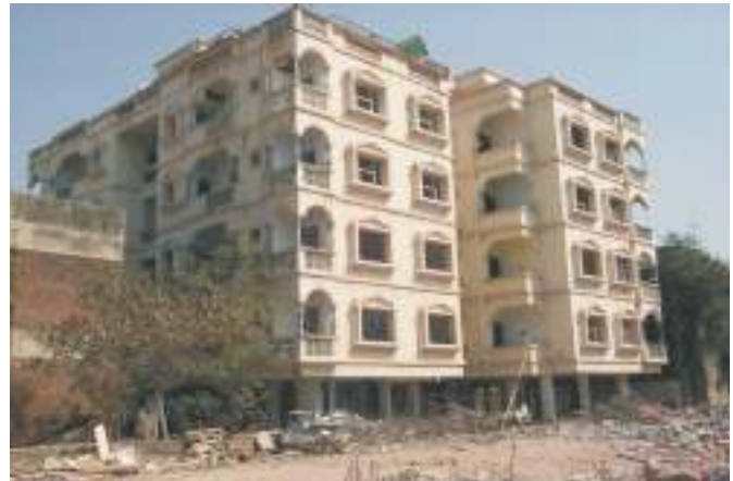
Fig. 10. A block of damaged reinforced concrete frame buildings in Ahmedabad with open first storey and brick masonry infills.
