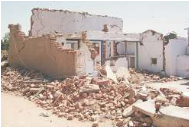
Fig. 6. Destruction of heavy stone masonry walls that had no reinforcement and were not tied to each other.
