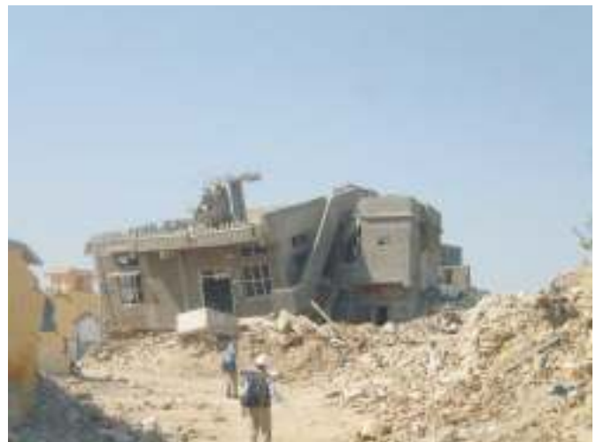
Fig. 8. A scene of destroyed load bearing masonry buildings in the town of Anjar.
