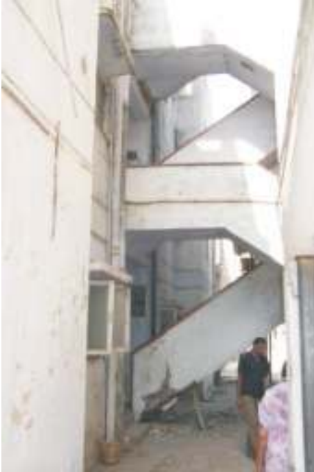
Fig. 22. The staircase interconnecting the two buildings in Fig. 20 allowed the building on the right to be supported by the building on the left.
