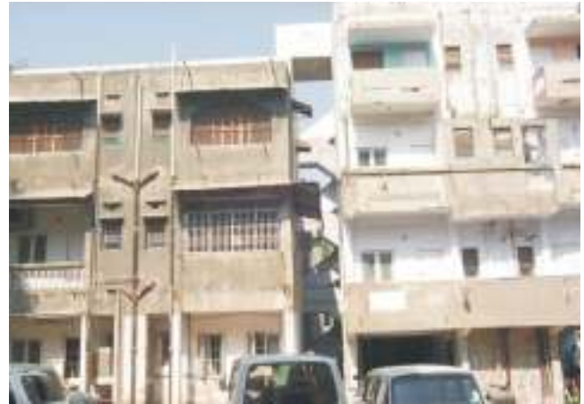
Fig. 20. Two adjoining buildings in Maninagar; the interconnecting staircase allowed the building on the left to support the building on the right.
