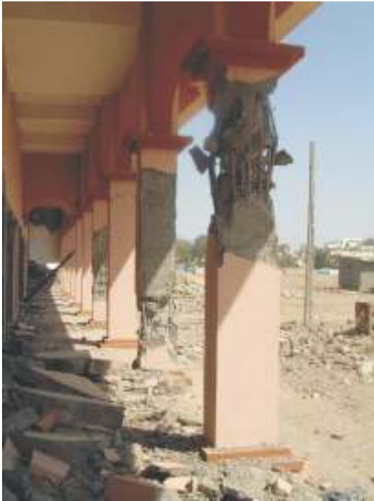
Fig 19. Failure of column through plastic hinging and buckling of longitudinal reinforcement due to loss of concrete cover and insufficient hoop reinforcement.
