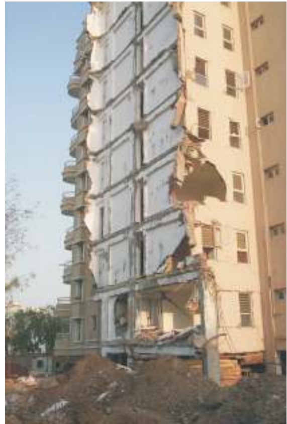
Fig. 13. One wing of the Shikhara building detached itself from the building and collapsed.
