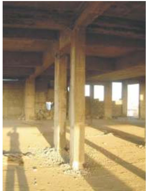
Fig. 29. Damage suffered by the columns in the partially completed upper floor of the Abha building in Bhuj.
