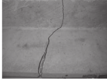
b) Crack Propagation Through the Deck
