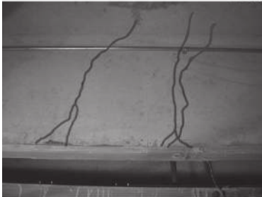
c) Crack Propagation Prior to Complete Peeling
