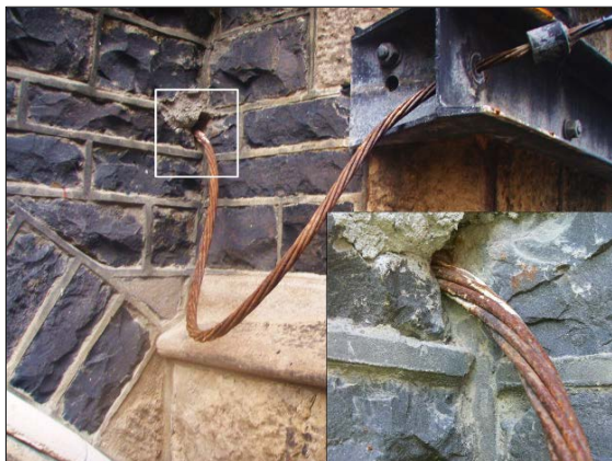
(a) Corrosion of PT steel (after tendon had been released to enable strengthening works)
