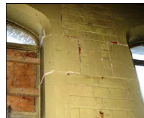
b) Differential movement between North Elevation buttresses and roof diaphragm
