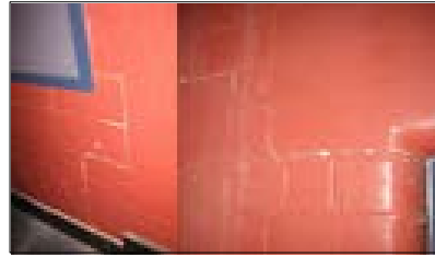
d) Ground floor - evidence of differential movement, spalling of mortar and residual displacement common at this level
