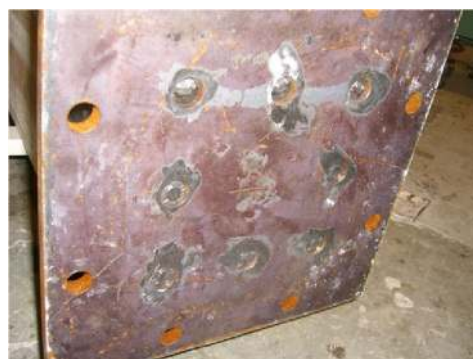
(c) Partial tensile failure of connection between LSB and column base joint
