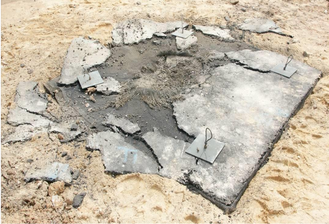
Figure 19. Damage of the multi-layer pavement after blast load with top layer AC in place
