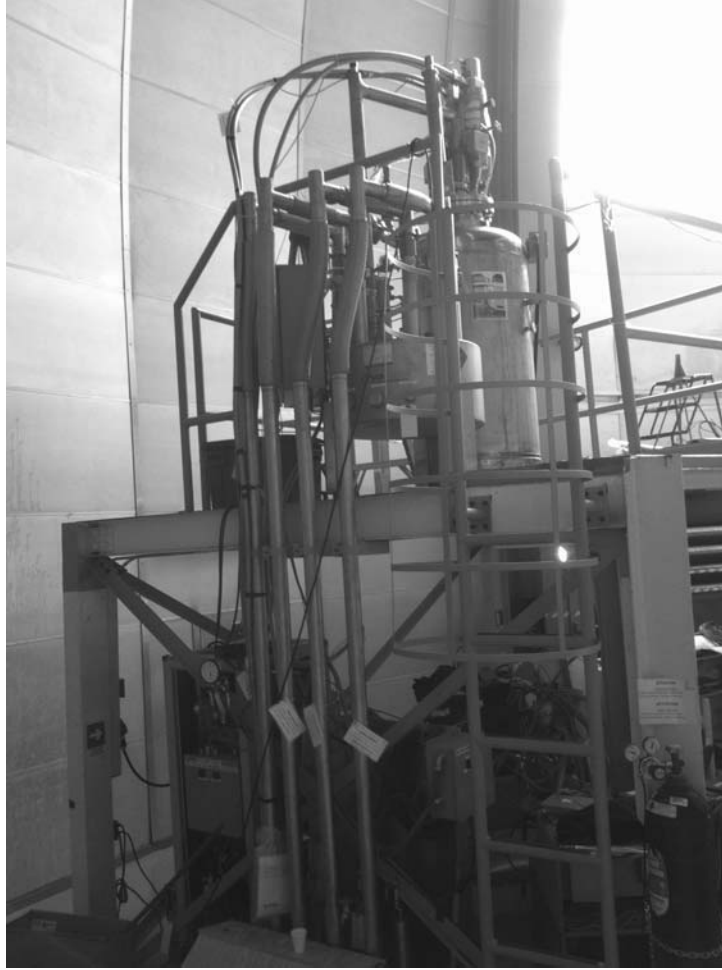
FIGURE 1. Process tank on the console room roof with valve box and transfer lines running to the Coudé room and to the telescope. The controls and instrumentation rack is located below the roof.
