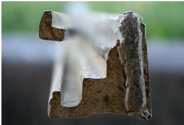
Figure 13. Typical separation of fatigue critical component from AM2 style mat joint.
