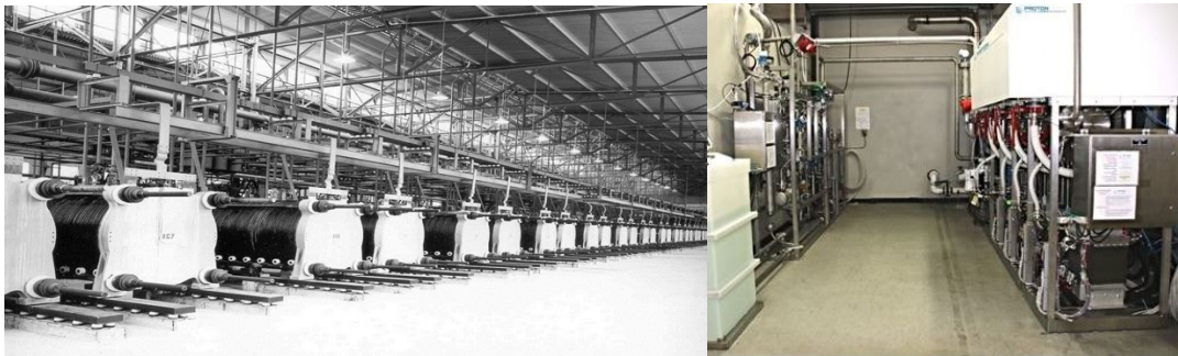
Figure 3: 135 MW KOH electrolyzer plant on left and 1 MW PEM system on right
