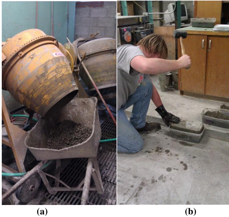
Figure A.1: Making pervious concrete by a) mixing the pervious concrete mixture in a drum concrete mixer and b) compacting each specimen with a concrete compactor form
