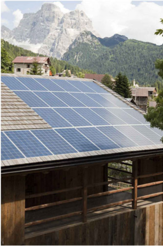
Figure 5. Energy self-sufficient tabià (retrofit), Selva di Cadore (Belluno), Italy, 2010. PV is part and parcel of the pre-existing wooden tilted roof. Design: EXiT. Picture by courtesy of the architects ©T. Cos.
