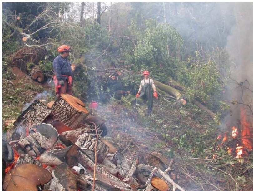
Figure 4 Host removal and burning as part of Phytophthora ramorum eradication efforts in southwestern Oregon. (Photos by A. Kanaskie, C. Brasier).
