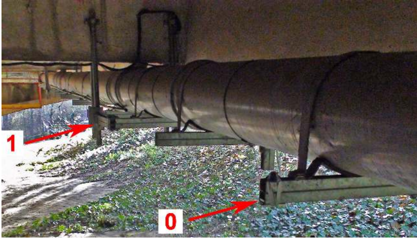
Figure 3. Locations of the sensors on the pipe.
