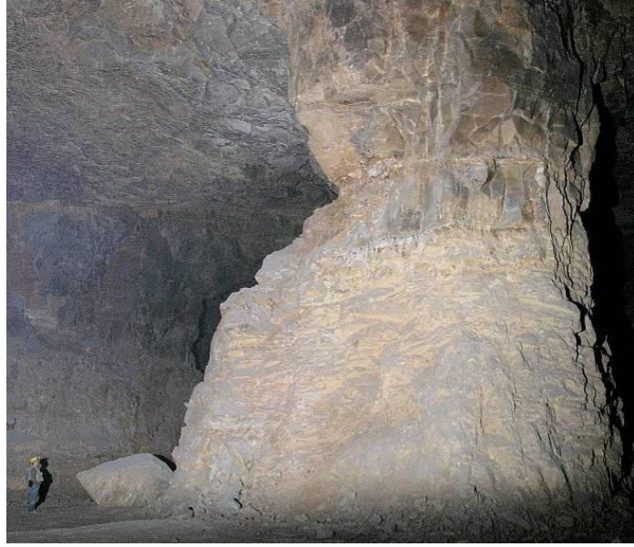
Figure 14. Rib failure related to large, angular discontinuities adjacent to a fault zone.
