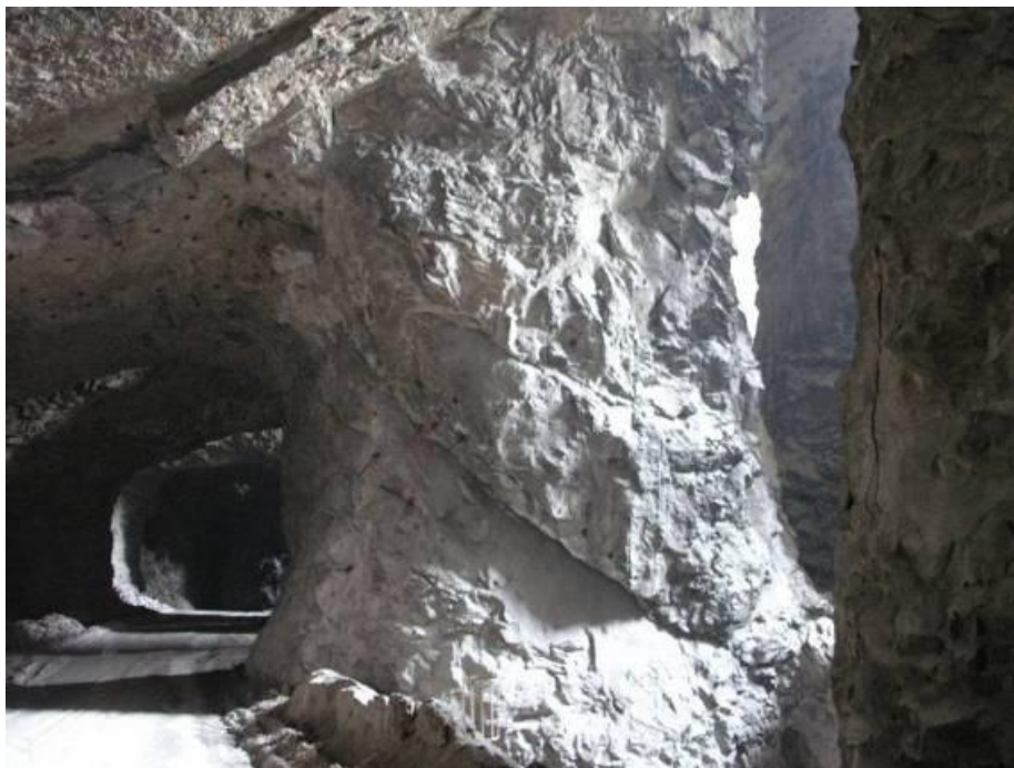
Figure 13. Example of a pillar that is bisected by a large, angular discontinuity.
