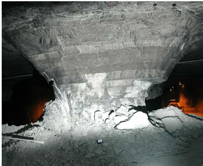
Figure 5. Pillar that had an original width-to-height ratio of 1.7, but failed by progressive spalling. Thin, weak beds are thought to have contributed to the failure. The average pillar stress was about 11% of the UCS prior to failure.
