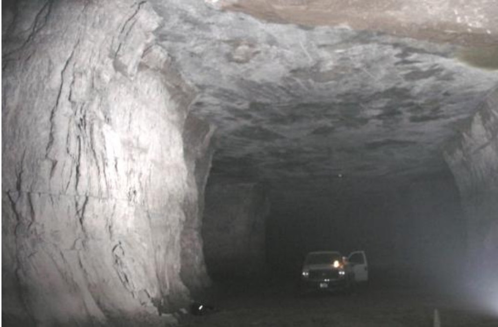
Figure 7. Example of rib spalling and resulting concave pillar ribs that can initiate when average pillar stress exceeds about 11% of the UCS.
