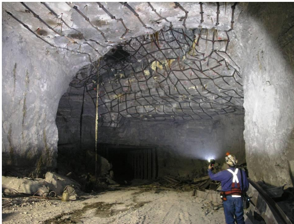
Figure 28. Bolts, straps, and injection grouting used to rehabilitate the roof at the site of a major roof fall.
