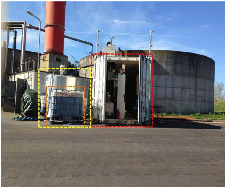
Figure 1. Impression of the pilot plant. The open container contained the selector and accumulator bioreactor (red bracket). In the front, there is an IBC sedimentation tank (orange bracket). Behind the sedimentation tank, the influent buffer vessel was located (yellow bracket). (Image by Michel Mulders.)
