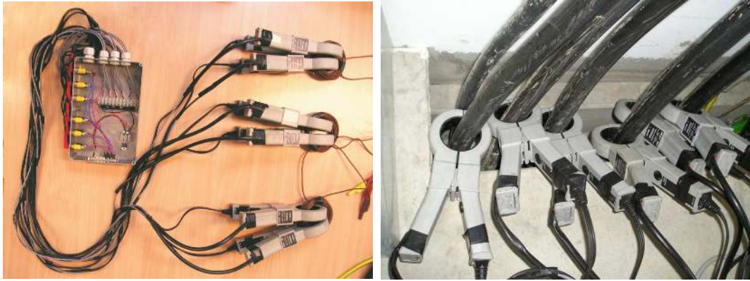
Figure 3.6. Current clamps with power supply unit(left), in real measurement (right)
