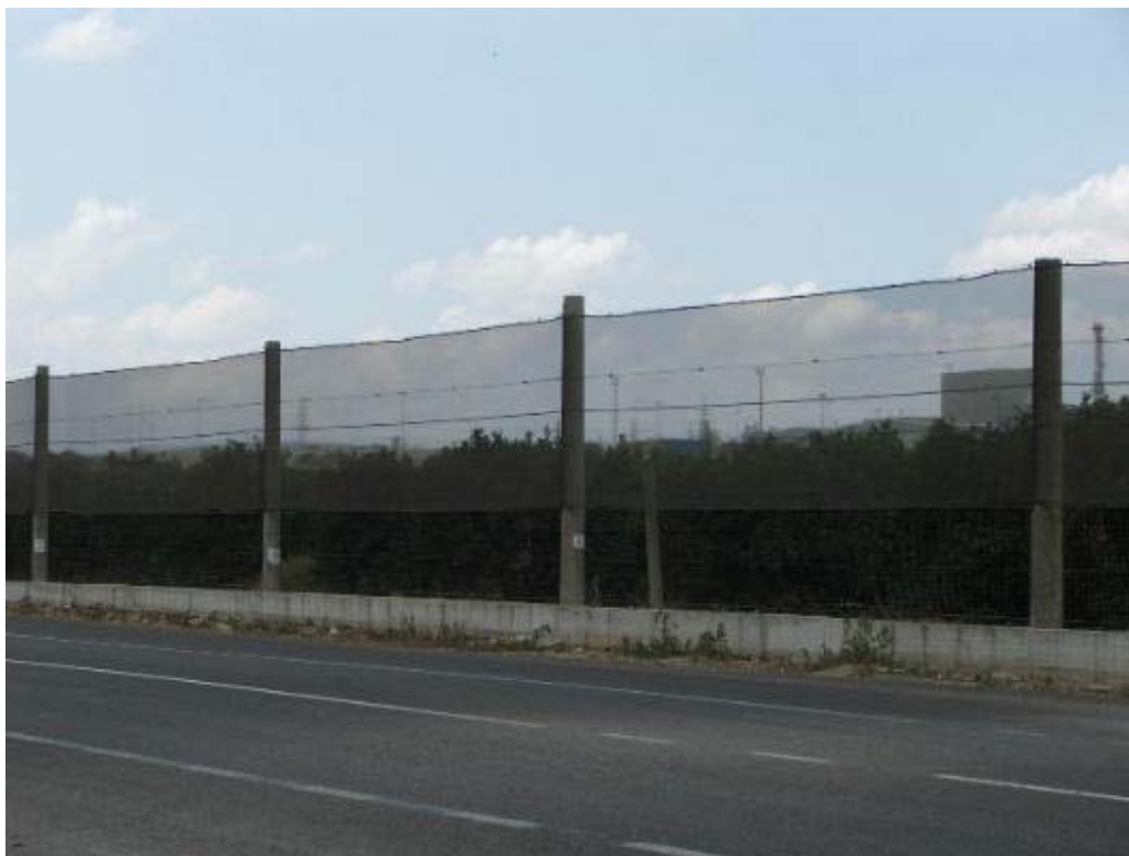
Figure 4. Windbreak net supported by a concrete structure in southern Italy.
