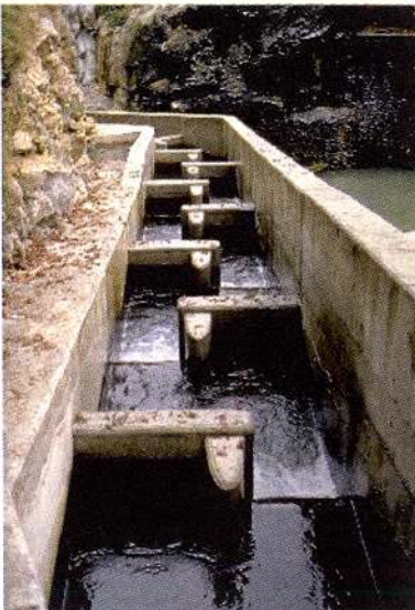
Photo 4: Small "plunging flow" salmonid fish pass at Cau dam (Gave d'Ossau, Atlantic Pyrenees).
