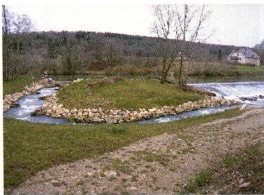
Photo 14: General view of the natural bypass channel at Chatillon sur Lison weir (river Loue).
