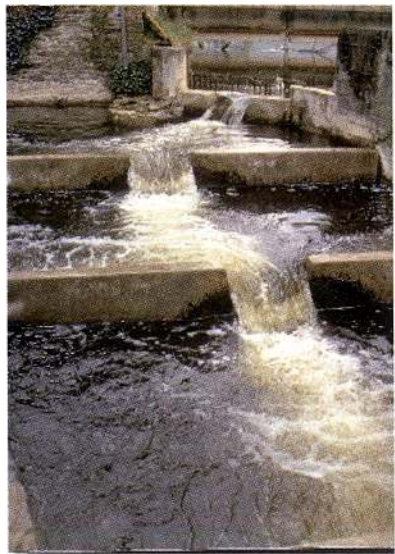
Photo 5: Semi-circular notch fishpass at the Hom dam, on the river Orne (Normandy).
