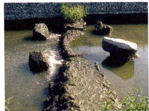
Photo 13: Detail of the V-shaped weir at the fishway at Sambeck dam on the river Meuse (Netherlands).
