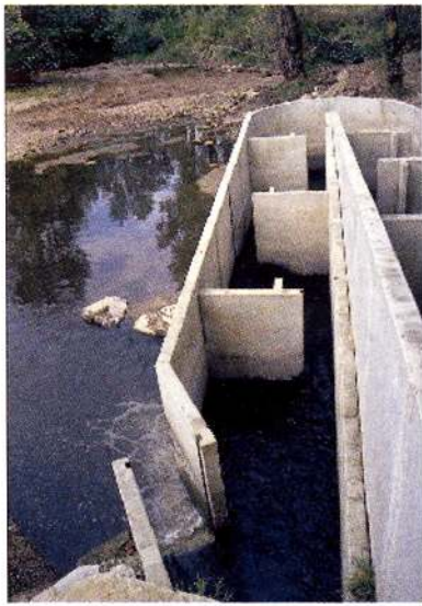
Photo 6: Deep lateral side notch and submerged orifice fish pass (Vézère river).
