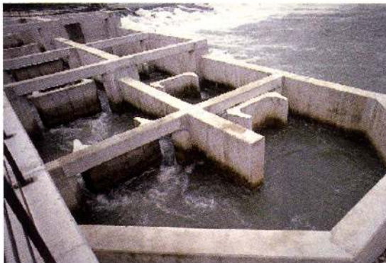
Photo 10: Chamfered angles in a change of direction pool in a large paired vertical slot fishway (Puyoo weir, river Gave de Pau).
