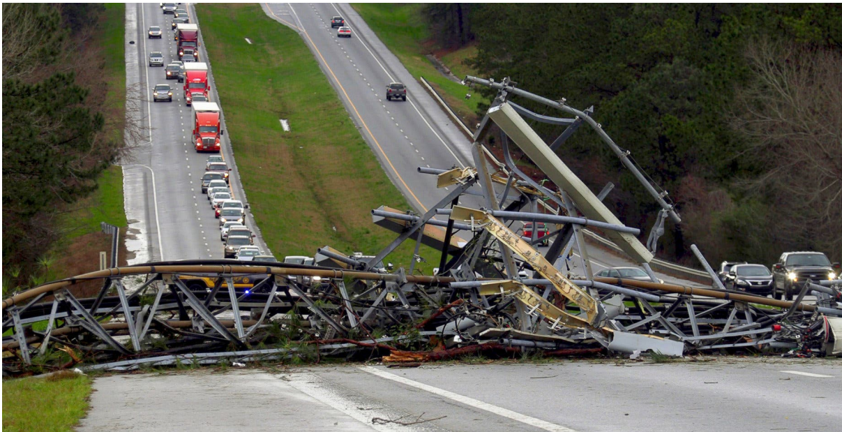
FIGURE 1. Disaster-struck cell tower [14].
