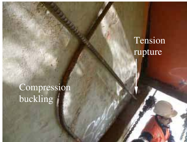
Figure 145. Photo. X-braces damage in south abutment of Pichibudis bridge.
