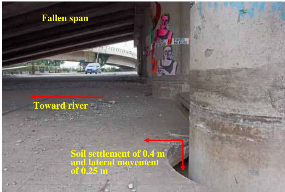
Figure 213. Photo. Settlement and lateral ground movement of interior pier at northeast end of Llacolen bridge.
