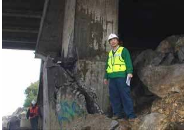
Figure 68. Photo. Shear failure in upstream column at northern end of Juan Pablo II bridge.
