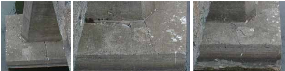
Figure 139. Photo. Cracks in pile caps of Biobío River bridge.
