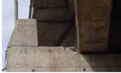
Figure 35. Photo. Close-up of damage to exit ramp from westbound Independencia bridge.
