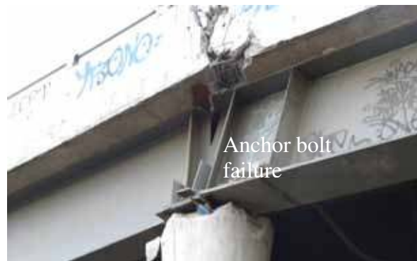
Figure 112. Photo. Damage to anchor bolts on Quilicura railway overcrossing.
