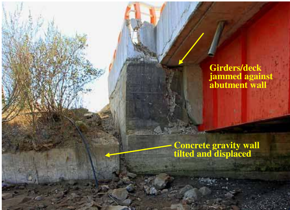
Figure 206. Photo. Abutment and girders shoved into each other and deck at the northwest abutment of the Raqui 1 bridge.
