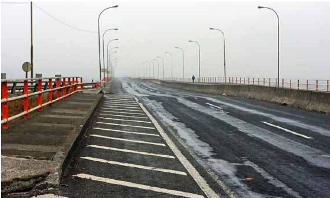
Figure 220. Photo. Roadway settlement due to settlement of mainline pier foundations for Juan Pablo II Bridge.
