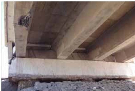
Figure 37. Photo. Bottom flange damage to Chada bridge.
