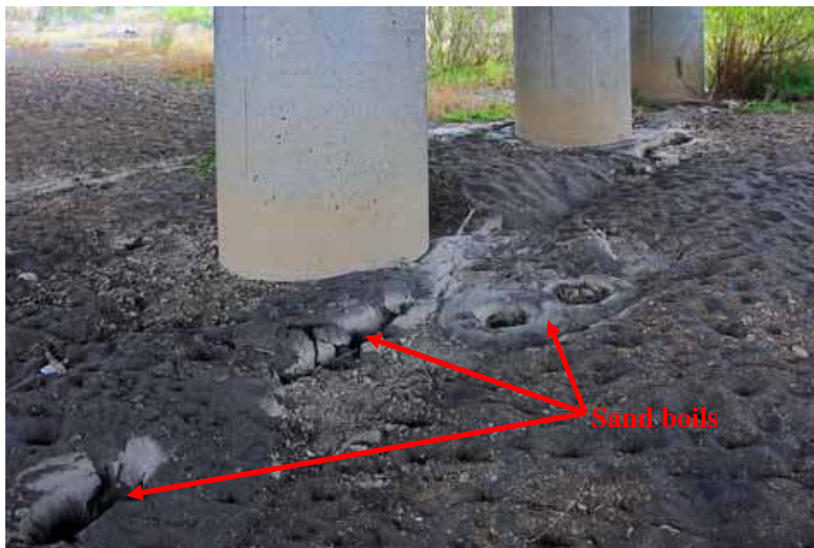
Figure 195. Photo. Sand boils at southwest end of Llacolen bridge.
