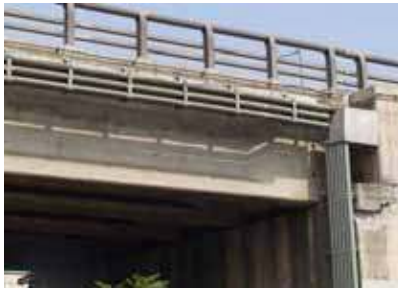
Figure 29. Photo. Shear key damage at abutment of westbound Independencia bridge.
