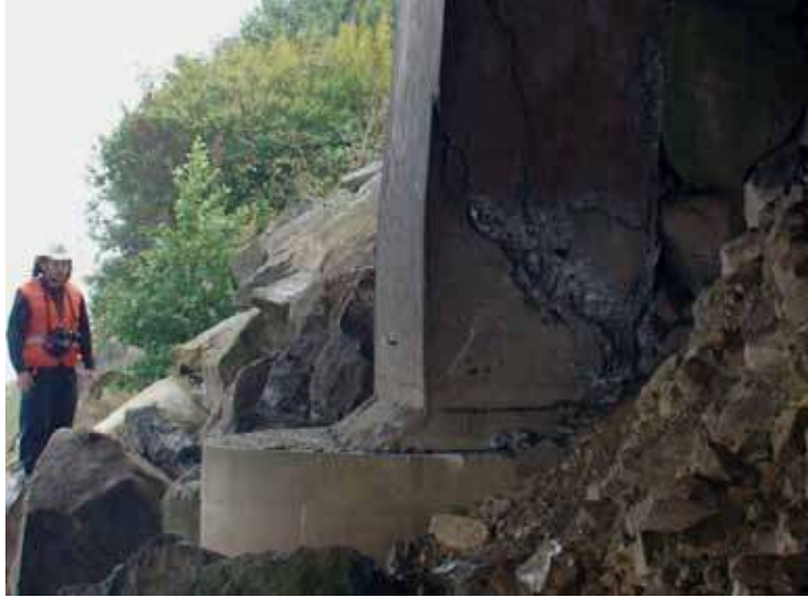
Figure 71. Photo. Shear failure in downstream column at northern end of Juan Pablo II bridge.
