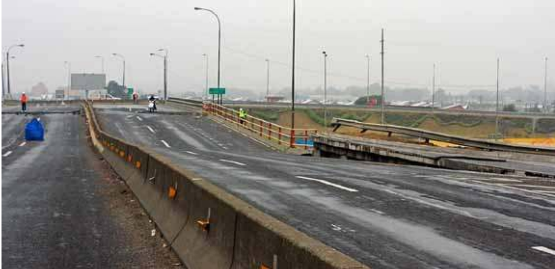
Figure 219. Photo. Roadway settlement due to settlement of approach structure pier foundations for Juan Pablo II bridge.
