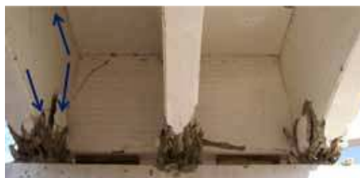
Figure 184. Photo. Longitudinal and vertical seismic forces in haunches at pier 3 of Maipú River bridge.
