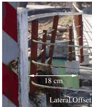
Figure 144. Photo. Offset in handrail on south abutment of Pichibudis bridge.
