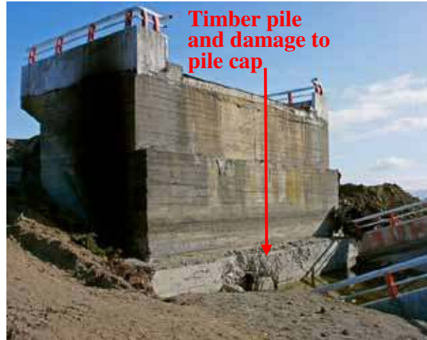
Figure 238. Photo. Overview of damage to south abutment of Tubul bridge.
