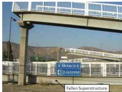
Figure 160. Photo. Damaged Route 5 pedestrian bridge.
