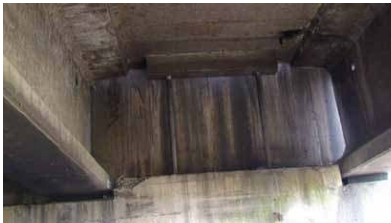
Figure 58. Photo. Spalling of shear key at southwest abutment of Llacolen bridge.
