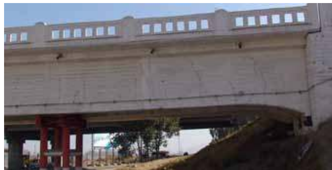
Figure 183. Photo. Shear cracks at span 1 of Maipú River bridge.
