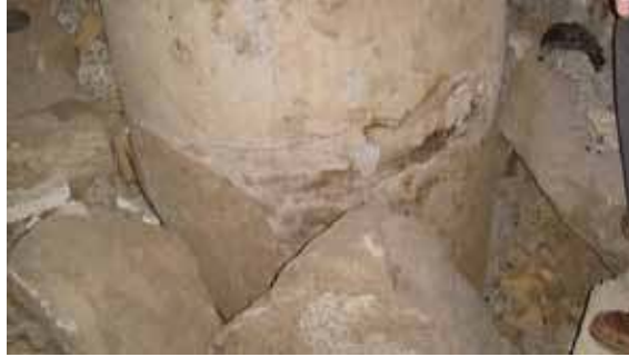
Figure 46. Photo. Flexural cracks at the level of rip rap on eastern approach to Llacolen bridge.
