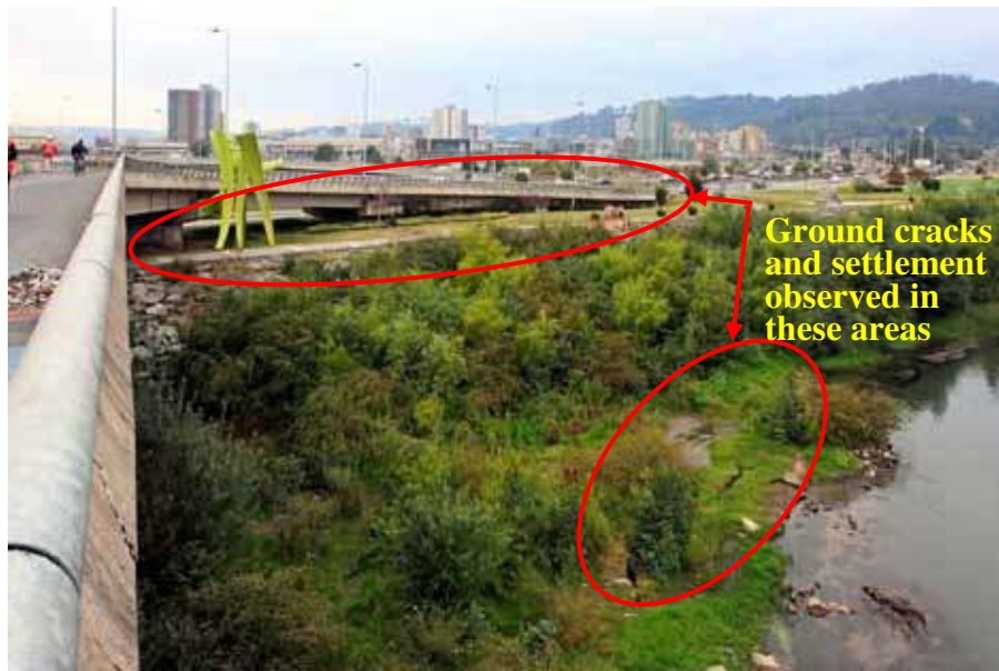
Figure 210. Photo. Evidence of slope instability due to liquefaction at northeast abutment and approaches of Llacolen bridge.
