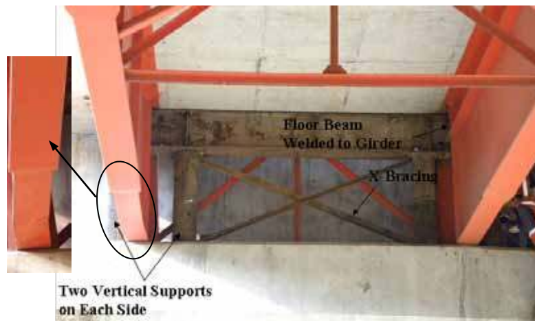
Figure 128. Photo. Temporary repair at northeast abutment of Cardenal Raúl Silva Henríquez bridge
