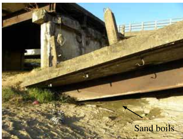
Figure 80. Photo. Sand boils near collapsed span in west Ramadillas bridge.
