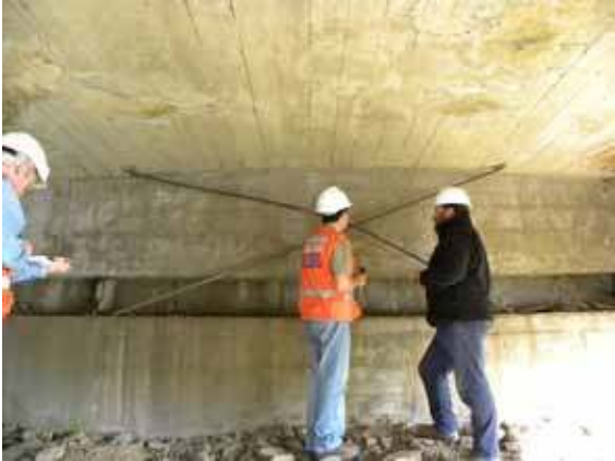
Figure 154. Photo. Damage to rebar X-brace system on north abutment of El Bar bridge.
