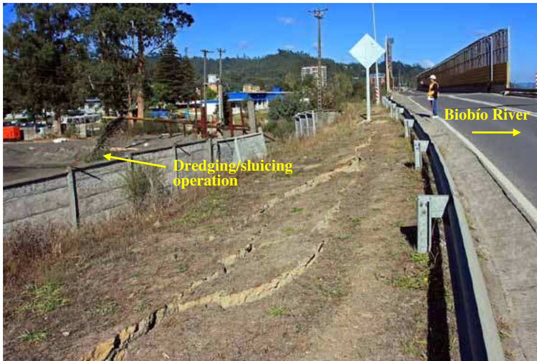
Figure 229. Photo. La Mochita bridge north approach fill and edge of dredging pit.
