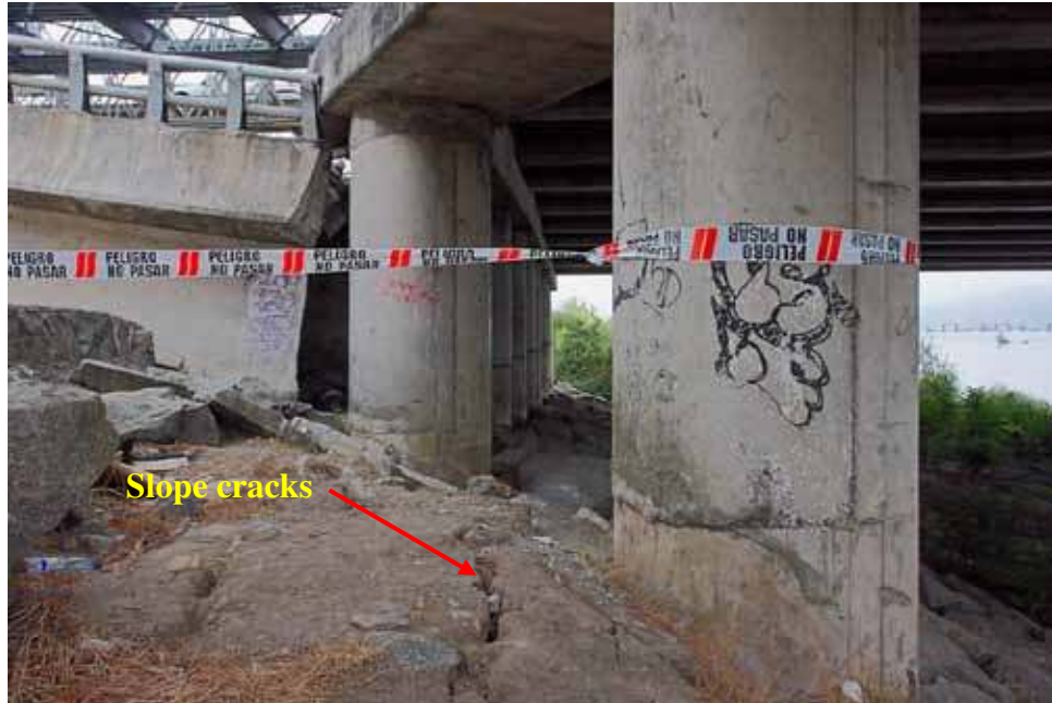
Figure 214. Photo. Lateral ground and foundation movement at interior pier and fallen span at northeast end of Llacolen bridge.
