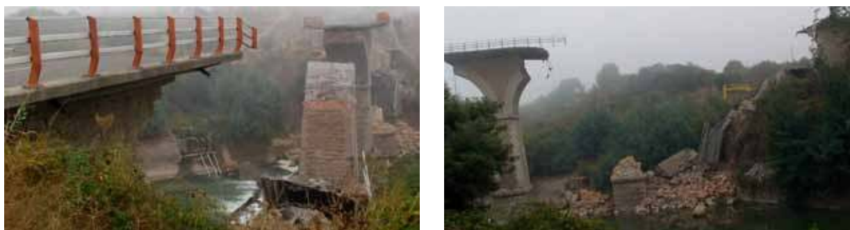
Figure 166. Photo. Close-up view of collapsed bridge at Claro River.
