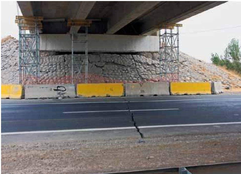
Figure 187. Photo. East abutment of Chada structure showing large pavement crack directly below bridge centerline.
