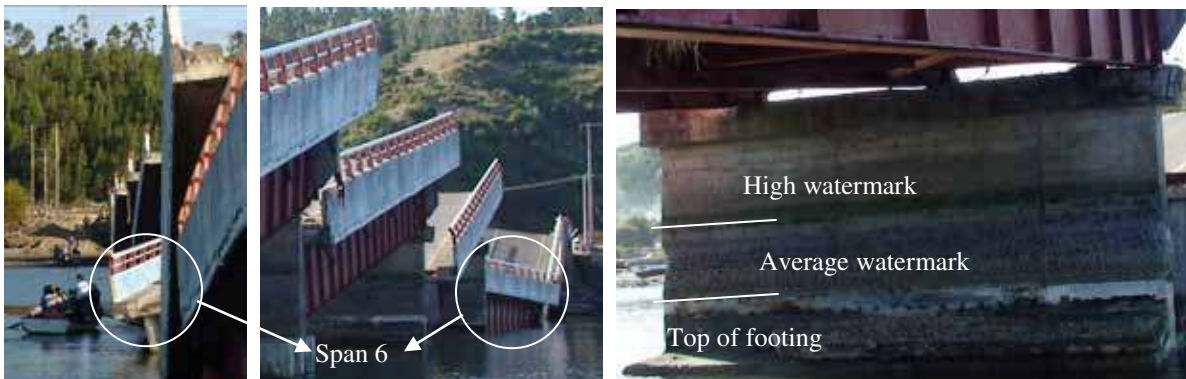
Figure 117. Photo. Span 6 of Tubul bridge, unseated at north end during an aftershock.
