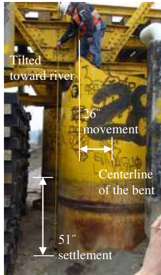
Figure 177. Photo. Settlement and tilting of bent on Chepe railroad bridge.
