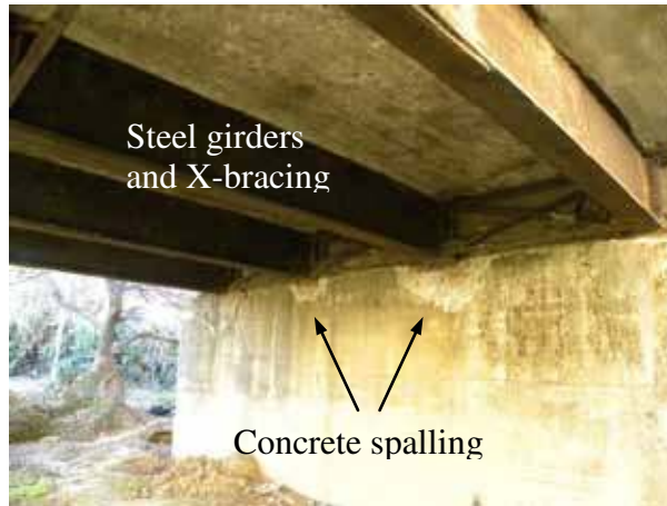
Figure 78. Photo. Abutment damage beneath west Ramadillas bridge.
