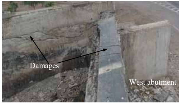
Figure 101. Photo. Back wall and wing wall damage at west abutment of Romero bridge.
