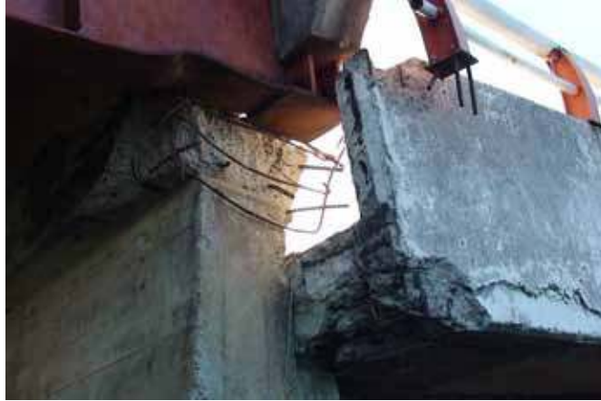
Figure 118. Photo. Bottom flange buckling and concrete spalling on Tubul bridge.
