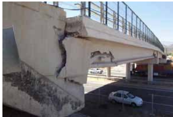
Figure 36. Photo. Curtain wall shear failure at abutment of Chada bridge.
