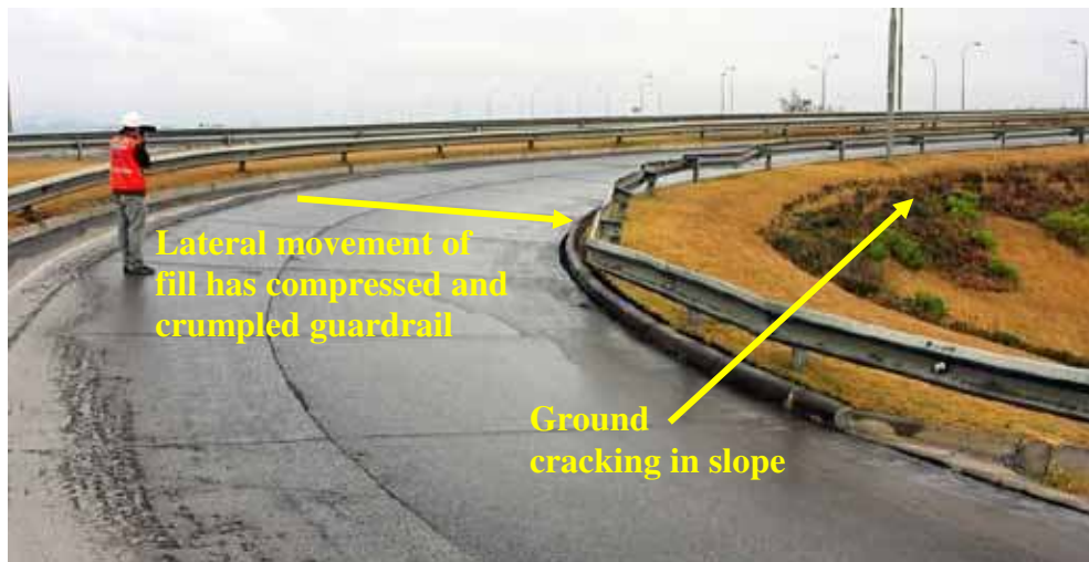
Figure 201. Photo. Lateral movement of fill in ramps at Juan Pablo II bridge.
