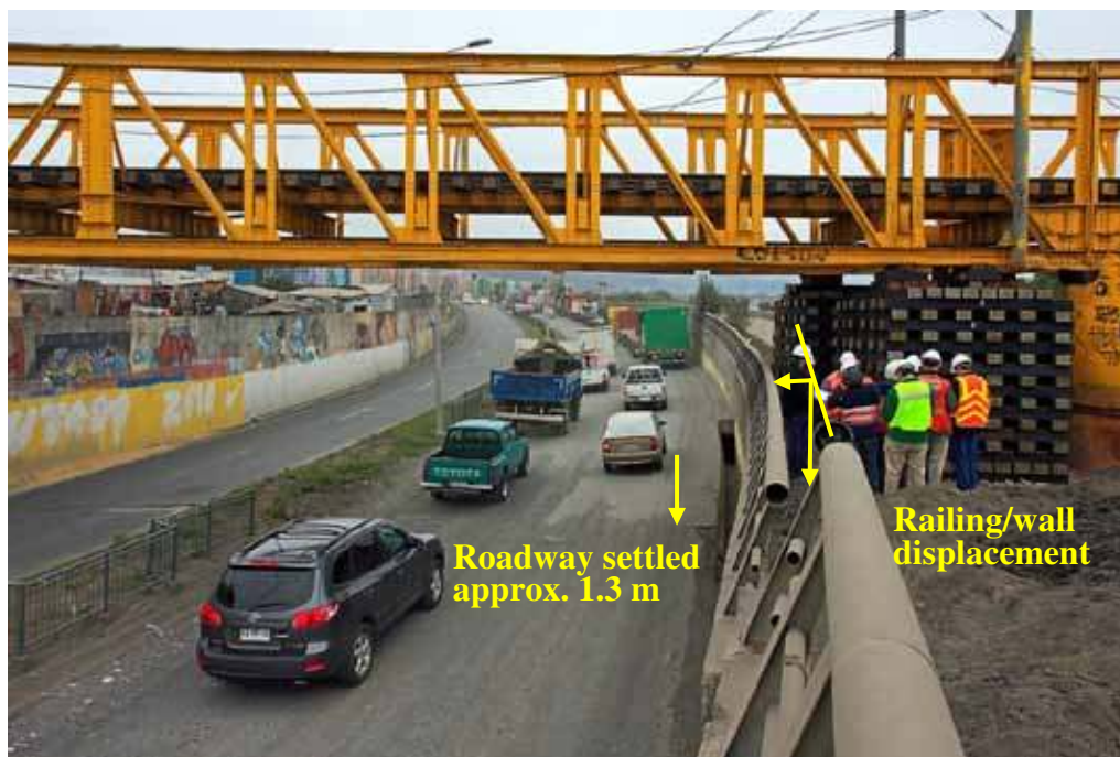
Figure 216. Photo. Wall settlement due to slope movement and instability caused by liquefaction at northwest end of Chepe railroad bridge.
