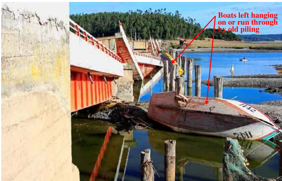
Figure 245. Photo. Tubul bridge with boats run through by old timber pilings.
