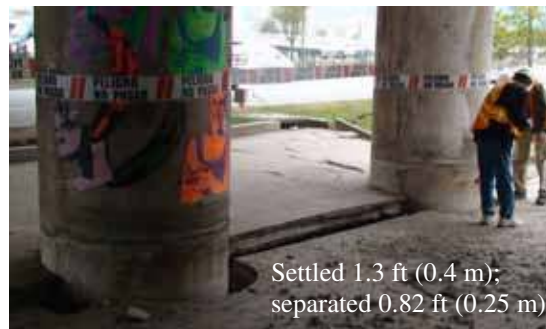
Figure 48. Photo. Ground settlement and lateral movement of eastern approach to Llacolen bridge.
