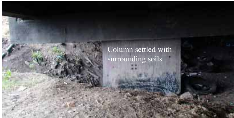
Figure 63. Photo. Column settlement under approach to Juan Pablo II bridge (cracks on far side).
