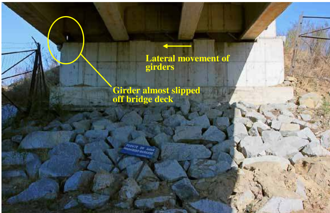
Figure 232. Photo. La Mochita bridge lateral bridge deck and girder at south abutment.
