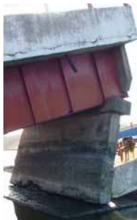
Figure 120. Photo. Tilting wall pier on Tubul bridge.
