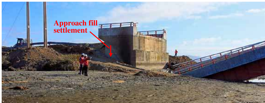
Figure 237. Photo. Settlement of fill beside the south abutment of Tubul bridge.
