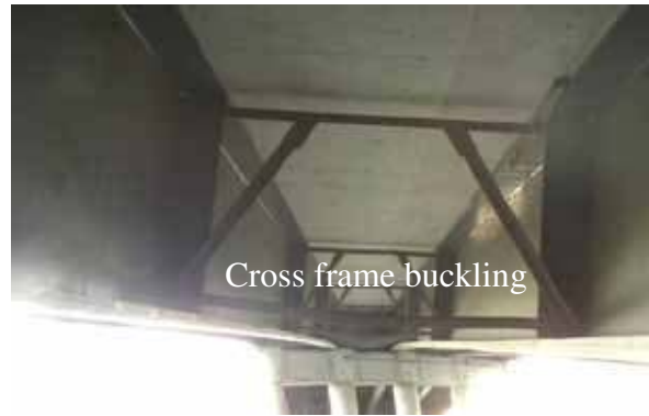
Figure 113. Photo. Damage to cross frame on Quilicura railway overcrossing.
