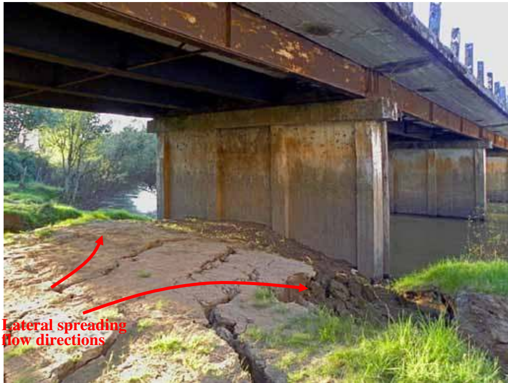
Figure 194. Photo. Lateral spreading and ground failure at old Ramadillas bridge.
