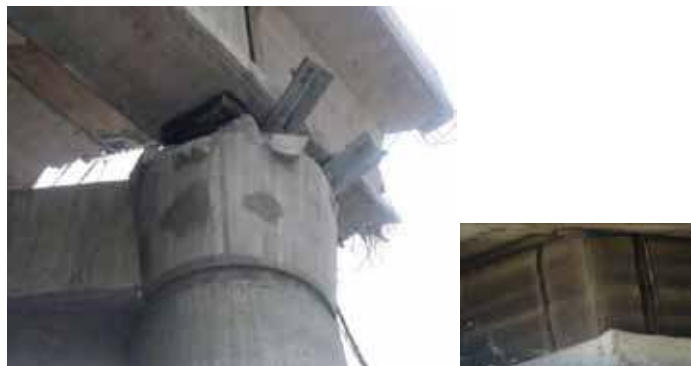
Figure 95. Photo. Displaced elastomeric bearing on Lo Echevers bridge.
