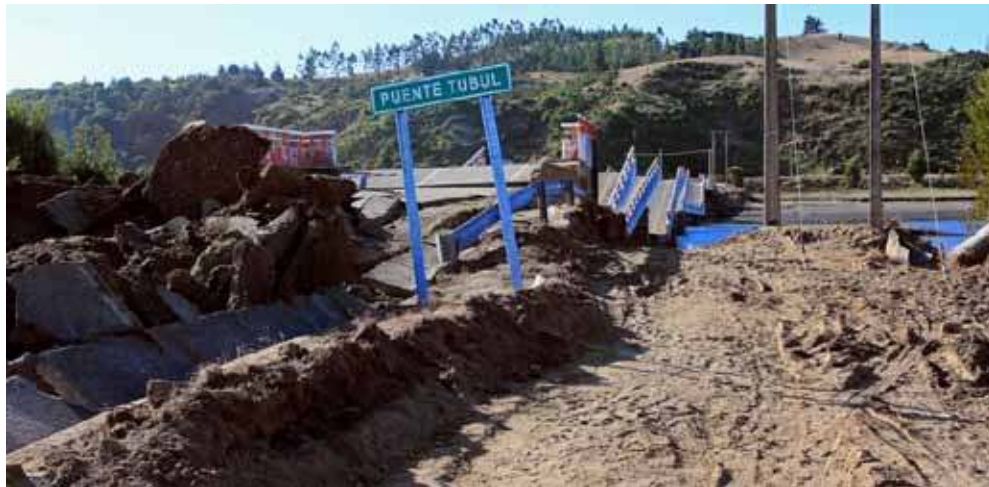
Figure 236. Photo. South approach fill damage and collapsed spans at Tubul Bridge.
