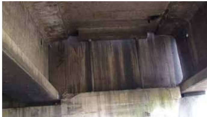
Figure 283. Photo. Exterior girder damage at west abutment of Llacolen bridge, concrete teeth.
