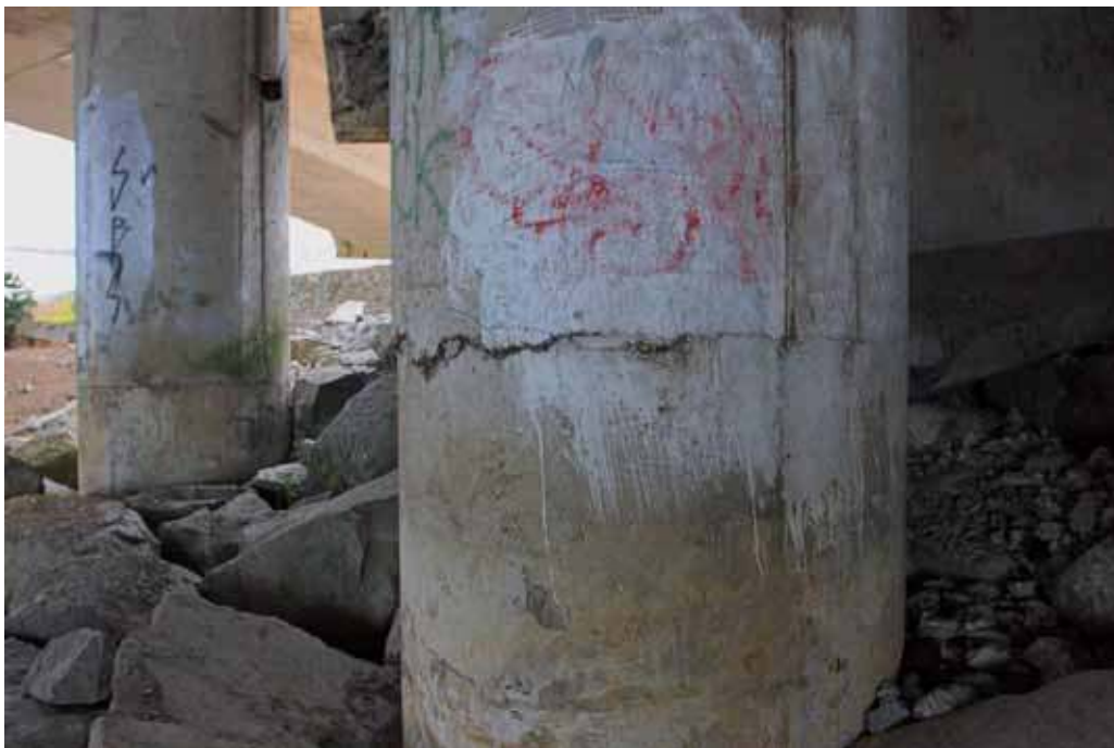
Figure 215. Photo. Close-up of cracked column at northeast end of Llacolen bridge.
