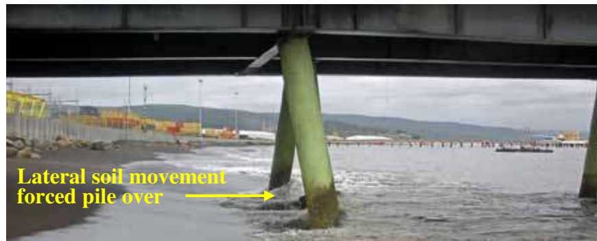
Figure 242. Photo. Puerto de Coronel Muelle foundation displacement and bending.
