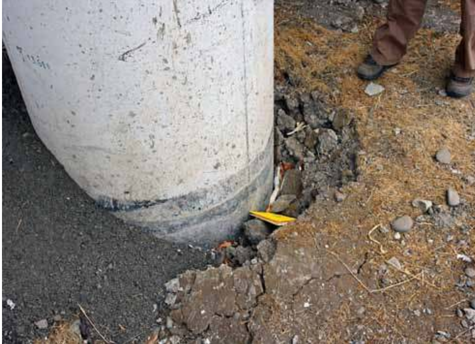
Figure 186. Photo. Interior pier of Chada structure with 5.8- to 7.8-inch (150- to 200-mm) gap in soil transverse to bridge centerline.
