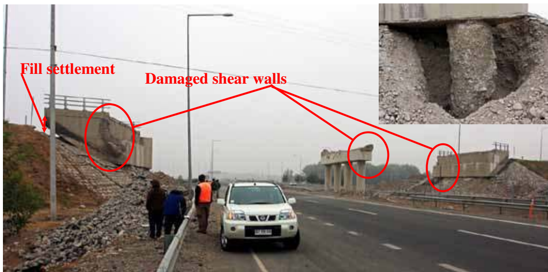
Figure 185. Photo. Damage at Romero bridge and shaft foundation supporting abutment (collapsed superstructure removed).
