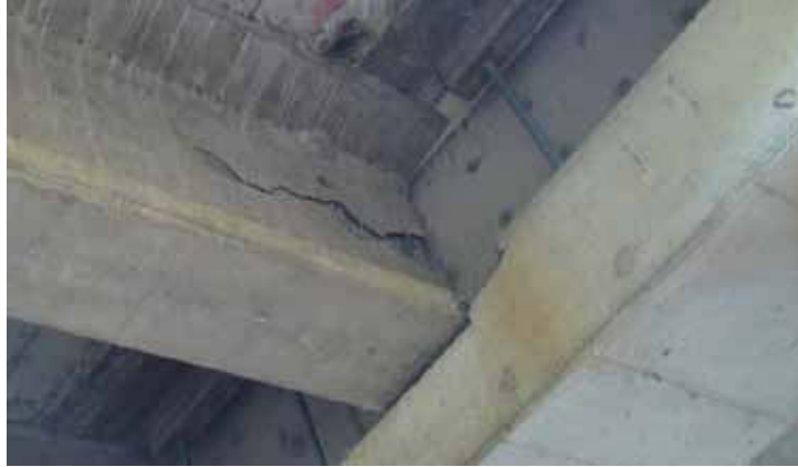
Figure 57. Photo. Horizontal crack in web of end girders at west end of Llacolen bridge.
