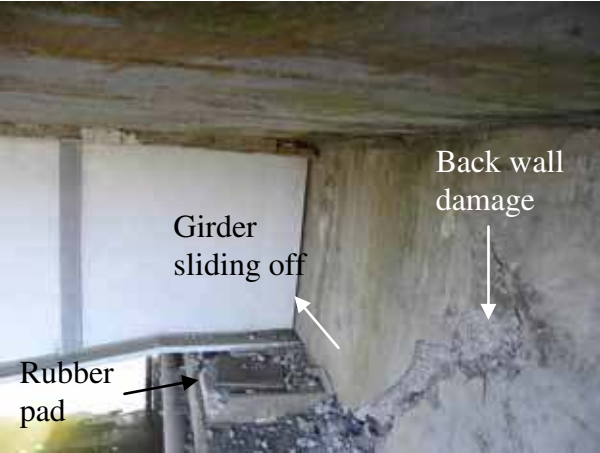
Figure 153. Photo. Damage at south abutment of El Bar bridge.
