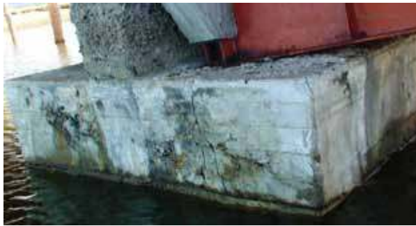
Figure 122. Photo. Crack in footing of Tubul bridge.
