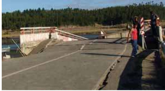
Figure 116. Photo. Buckling of pavement at north abutment of Tubul bridge.
