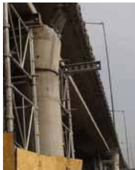
Figure 23. Photo. Damage to eastbound Independencia bridge.
