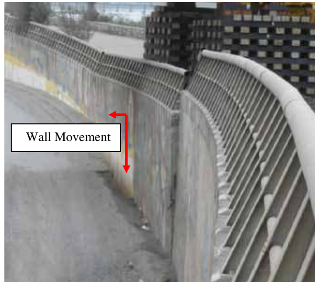
Figure 262. Photo. Wall movement near Chepe railroad bridge due to lateral spreading and settlement.
