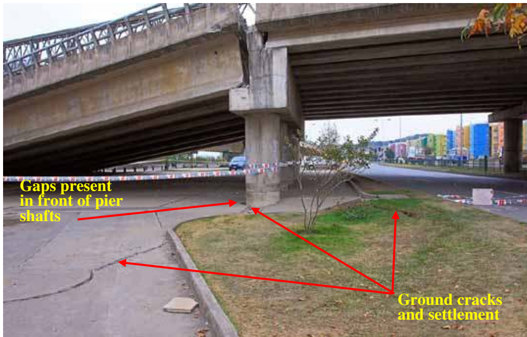
Figure 212. Photo. Settlement due to liquefaction-induced slope instability at northeast end of Llacolen bridge.
