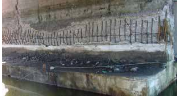
Figure 121. Photo. Spalling due to shear action and vertical crack in Tubul bridge.
