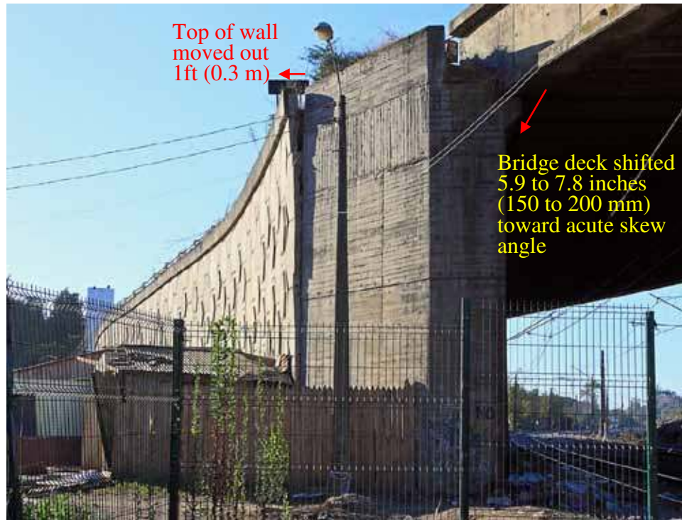
Figure 268. Photo. Wall corner tilting outward at wall site 28B.
