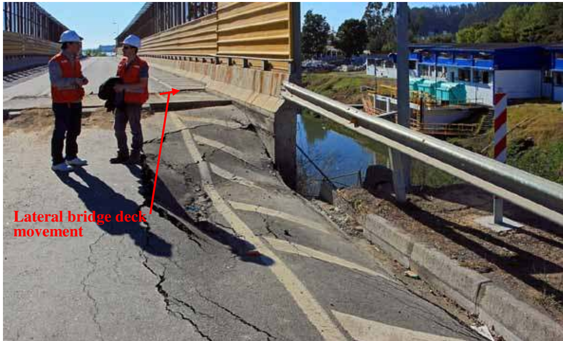
Figure 231. Photo. La Mochita bridge deck and girder lateral movement and approach fill settlement.
