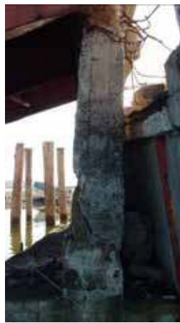
Figure 119. Photo. Shear crack in Tubul bridge.
