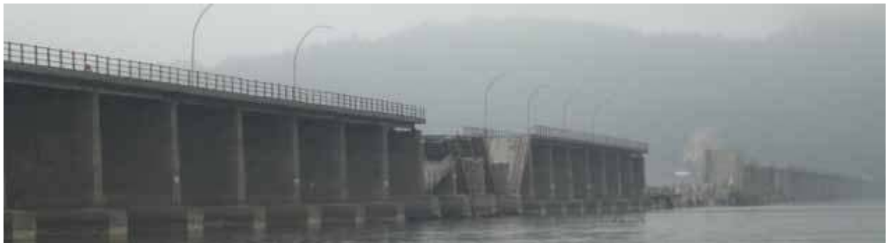
Figure 135. Photo. Collapsed spans in Biobío River bridge.
