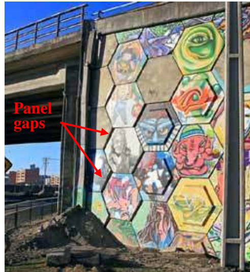
Figure 272. Photo. Differential settlement at wall site 28C.
