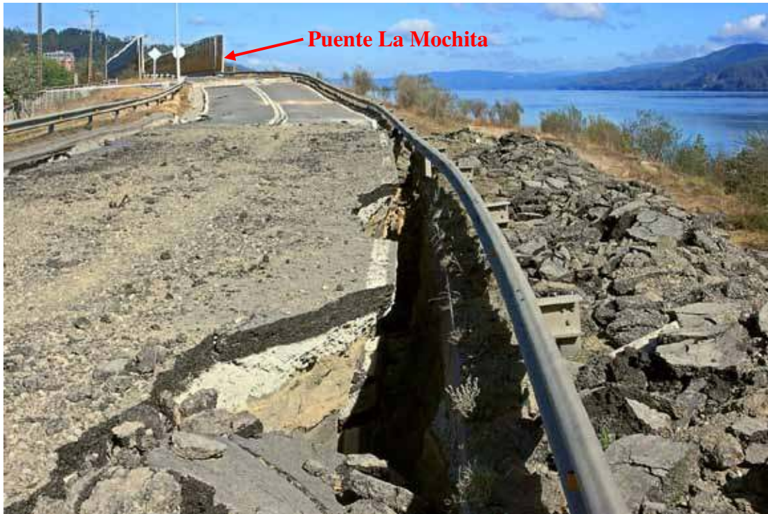
Figure 228. Photo. La Mochita bridge north approach fill liquefaction-induced ground failure.
