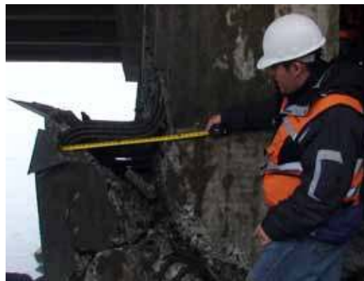
Figure 69. Photo. Front face of failure plane at northern end of Juan Pablo II bridge.
