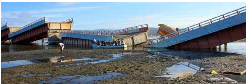
Figure 241. Photo. Tubul bridge collapsed spans and substructure.
