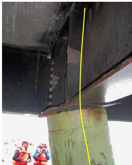
Figure 243. Photo. Close-up of Puerto de Coronel Muelle foundation displacement and bending.
