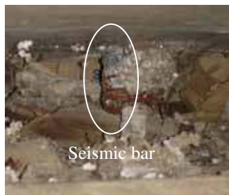
Figure 52. Photo. Seismic bar condition on westbound ramp to Llacolen bridge.
