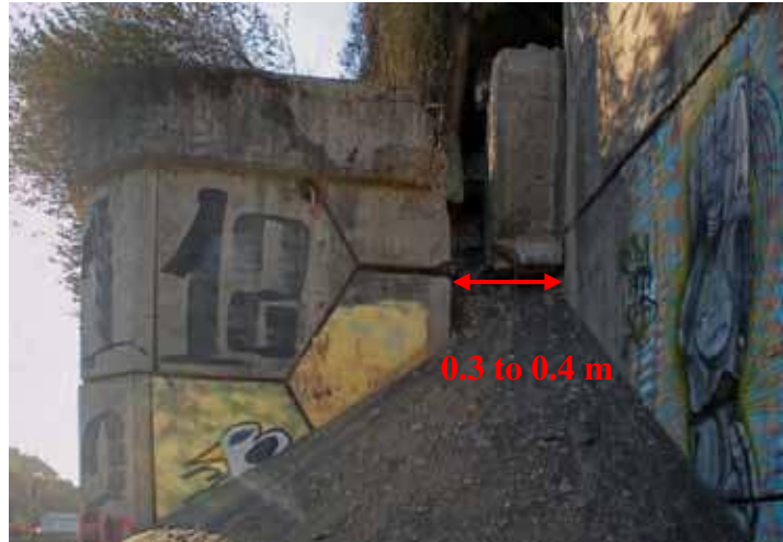
Figure 269. Photo. Lateral movement of lower wall top at wall site 28C.
