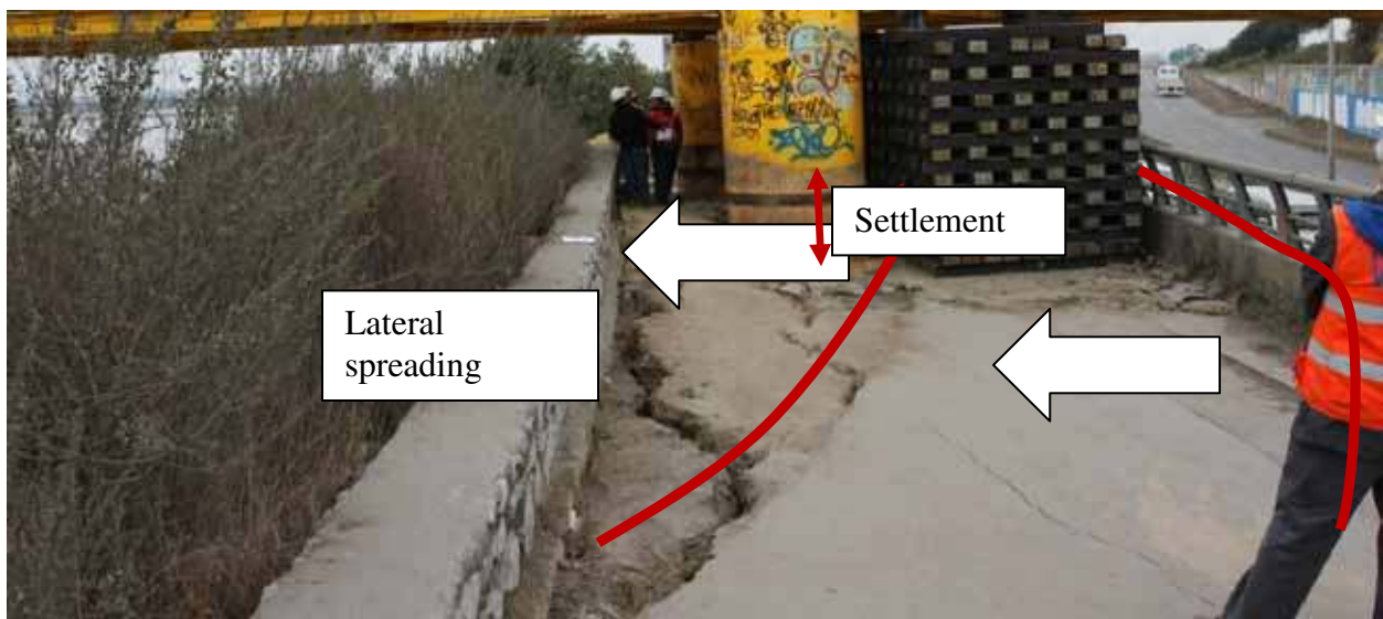
Figure 263. Photo. Wall settlement and rotation due to lateral spreading and settlement.
