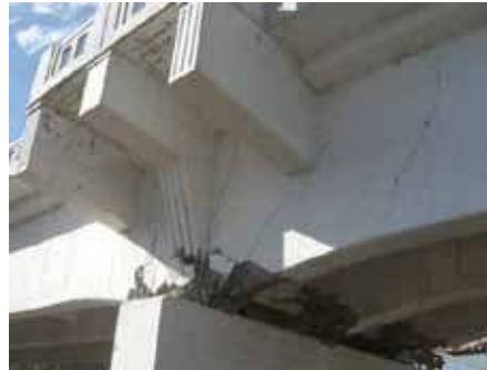
Figure 182. Photo. Crushing of haunches at pier 3 of Maipú River bridge.
