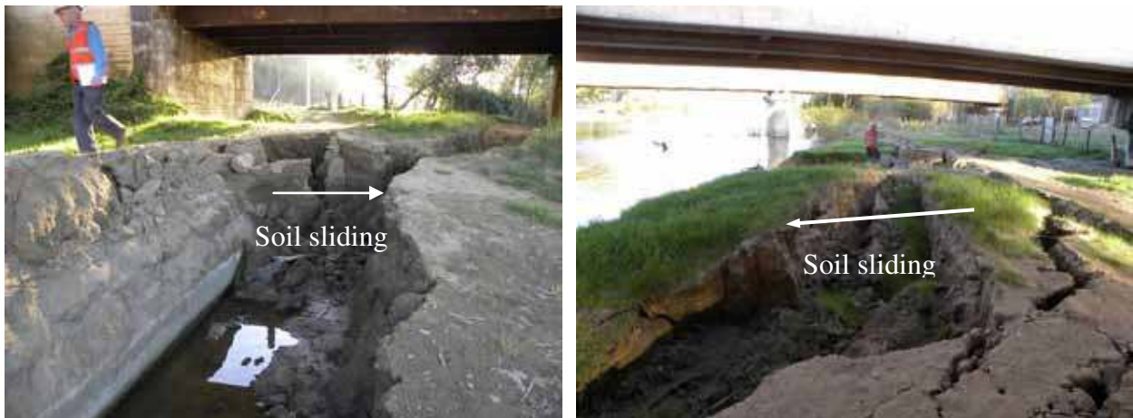
Figure 83. Photo. Block flow toward river due to liquefaction on south bank of Ramadillas bridges.
