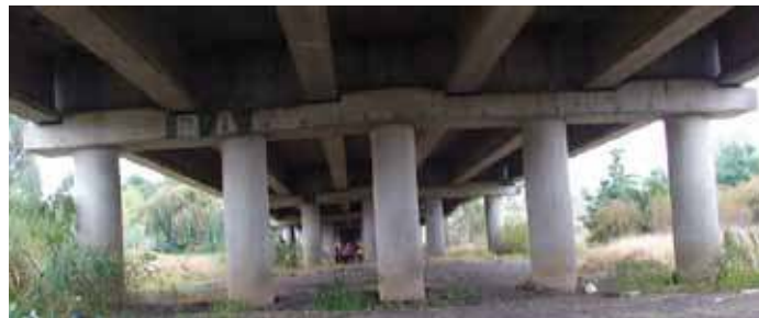
Figure 54. Photo. Columns with soil marks indicating ground settlement at west end of Llacolen bridge.
