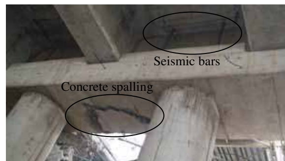
Figure 45. Photo. Concrete spalling beneath cap beam of eastern approach to Llacolen bridge.
