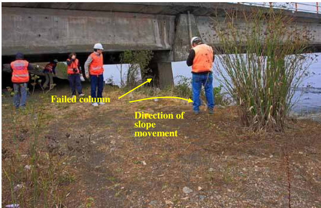
Figure 222. Photo. Damage to pier columns for mainline Juan Pablo II bridge.
