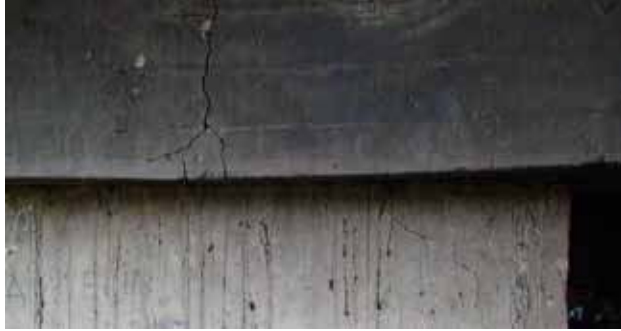
Figure 66. Photo. Cracks on far side of undamaged column under approach to Juan Pablo II bridge.
