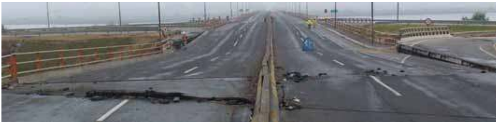
Figure 60. Photo. Southwest view of northern approach to Juan Pablo II bridge, facing Biobío River.
