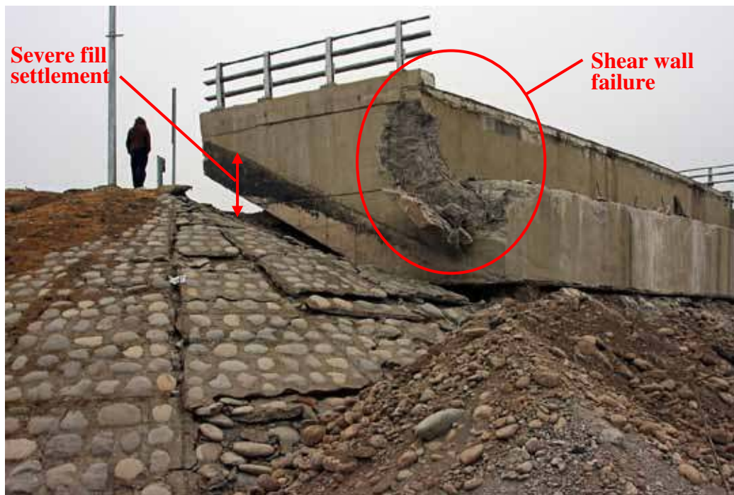
Figure 189. Photo. Fill slumping observed at Romero bridge.
