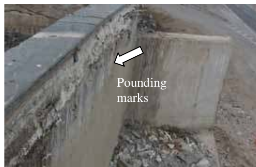
Figure 100. Photo. Pounding at west abutment of Romero bridge.
