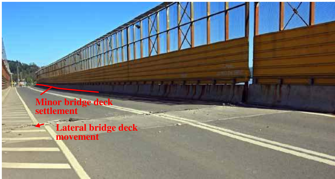
Figure 230. Photo. La Mochita bridge deck and girder lateral movement.
