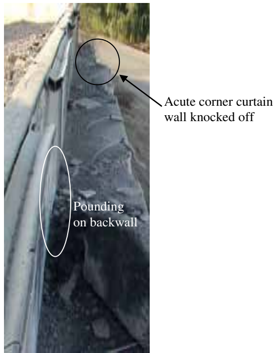
Figure 104. Photo. Damage at north abutment of Route 5 overcrossing at Hospital.
