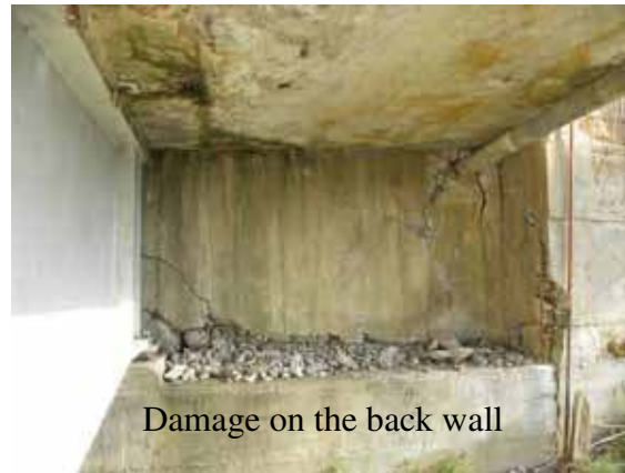
Figure 155. Photo. Damage to north abutment back wall of El Bar bridge.
