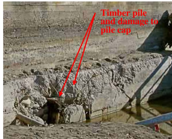
Figure 239. Photo. Close-up of exposed pile and pile cap damage on south abutment of Tubul bridge.
