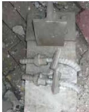
Figure 94. Photo. Failure of a steel stopper on Lo Echevers bridge.
