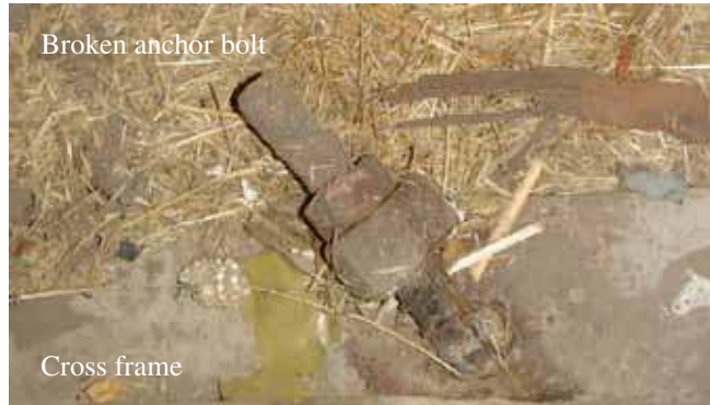
Figure 163. Photo. Anchor bolt failure (shear and pull out) on Route 5 pedestrian bridge.
