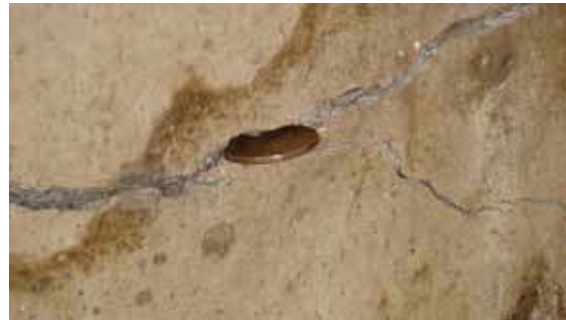
Figure 47. Photo. Close-up view of cracks at the level of rip rap on eastern approach to Llacolen bridge.
