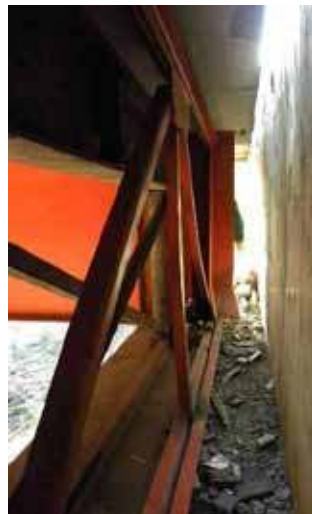
Figure 126. Photo. Cross frame buckling on Cardenal Raúl Silva Henríquez bridge.
