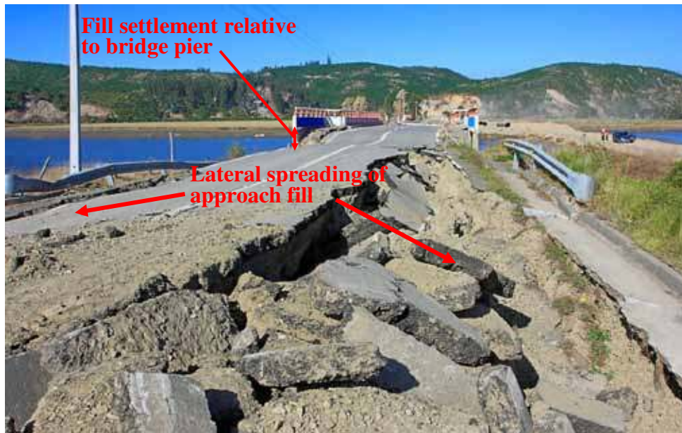
Figure 198. Photo. Lateral spreading and ground failure at Raqui 2 bridge.
