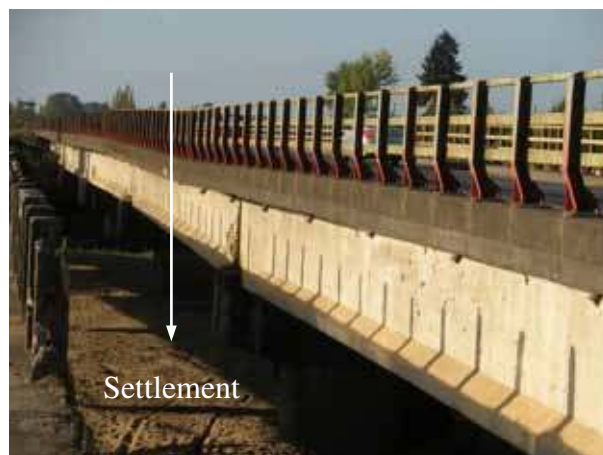
Figure 75. Photo. Deck misalignment under east Ramadillas bridge.
