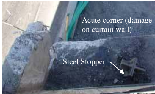
Figure 90. Photo. Acute corner of southwest abutment of Miraflores bridge.
