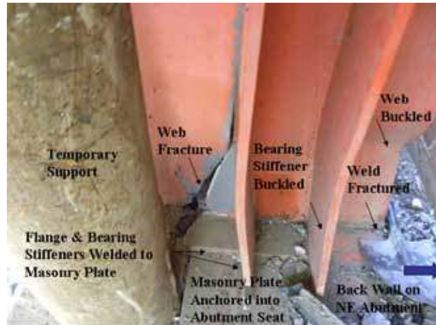
Figure 127. Photo. Girder damage at northeast abutment of Cardenal Raúl Silva Henríquez bridge.
