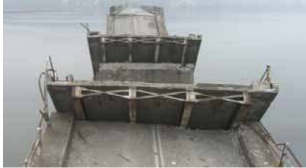
Figure 136. Photo. Unseated spans in Biobío River bridge.
