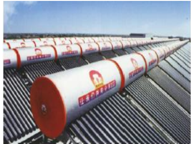
Fig. 7 SWH system installed on a rooftop [26]
