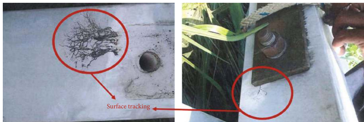
FIGURE 12: Surface tracking of PGFRP composite cross arm beams.
