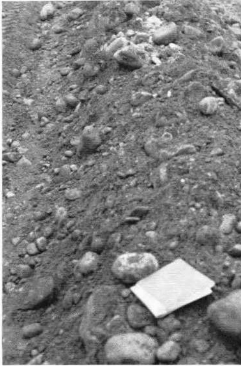
Fig. 47. Typical natural alluvial sand-gravel mixture meeting the gradation of Fig. 46. Thick zones of material of this general nature, used without processing, constitute good, self-healing and internally stable transitions
