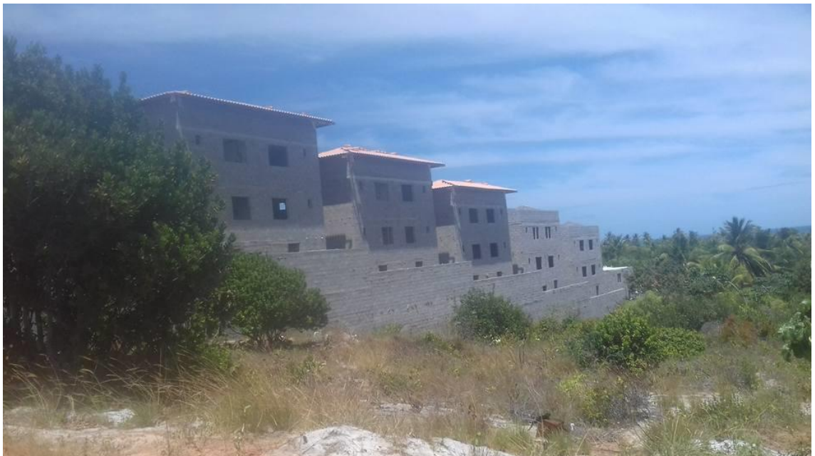
Photo 7-XIX: Illegal construction Source: Tony (17_I_1)
