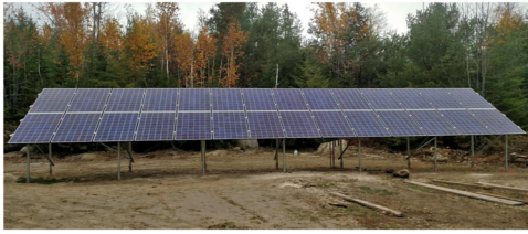
Fig. 12 Examined PV modules placed outdoor after the PID test is completed. The PV system consists of 28 modules distributed among two strings, each string comprising 14 modules.
