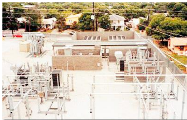
Figure 2.21: Image of BTB HVDC at Eagle Pass, U.S. (Courtesy: ABB)
