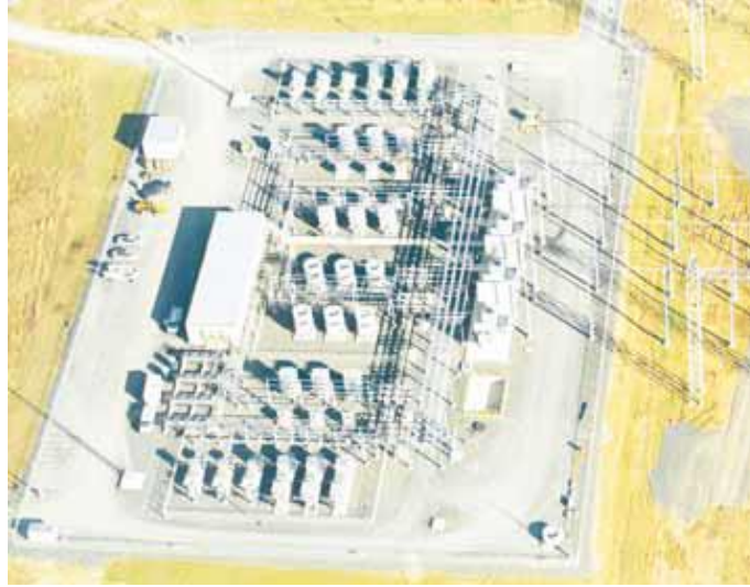
Figure 2.5: 500 kV, -145/+575 MVAR at Rawlings, Maryland, U.S. (Courtesy: ABB)
