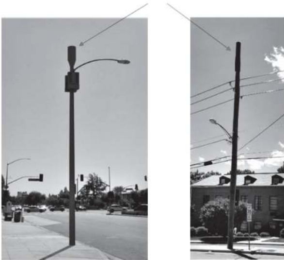
Microcell towers, usable in 5G and 5G IoT
