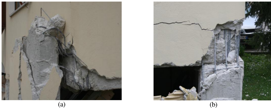
Figure 4. Damage highlights not properly treated casting surface (a, b) and absence of stirrups in the joint area (b) [15]
