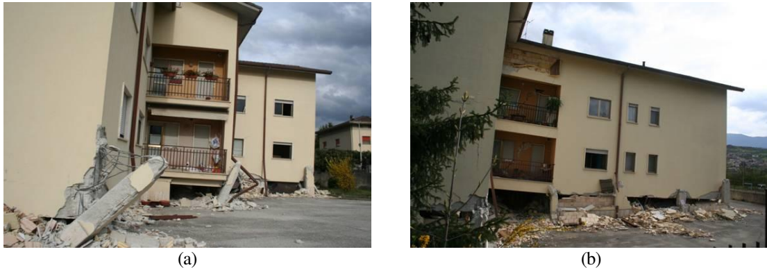
Figure 2 . Building collapse mechanism. Damage along South-East (a) and South-West (b) wings of the building [15]
