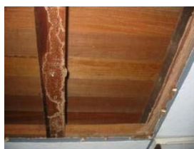
Termite infestation of ceiling Joist
