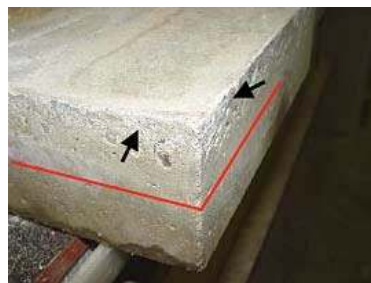
Figure 4.3 Concrete slab experiencing deterioration due to salt crystallization.
