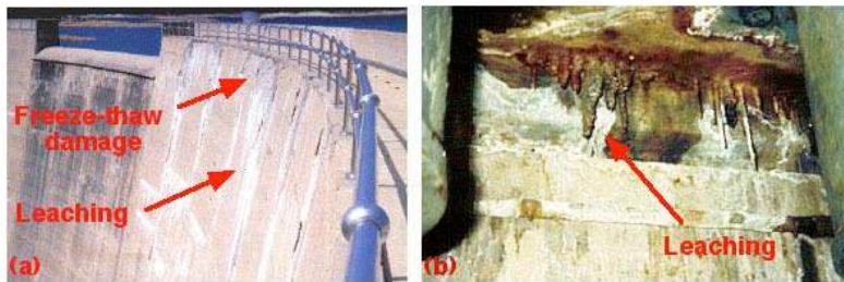
Figure 4.12 Examples of leaching of concrete: (a) dam with freeze-thaw damage and leaching, (b) nuclear power plant tendon gallery leaching.
