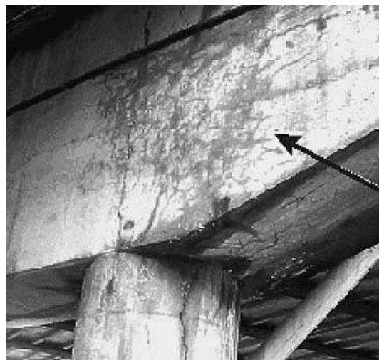
Figure 4.16 Cracking damage in a concrete structure due to DEF.
