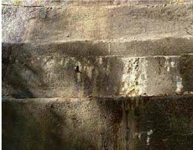
Figure 4.10 Efflorescence in water structure.
