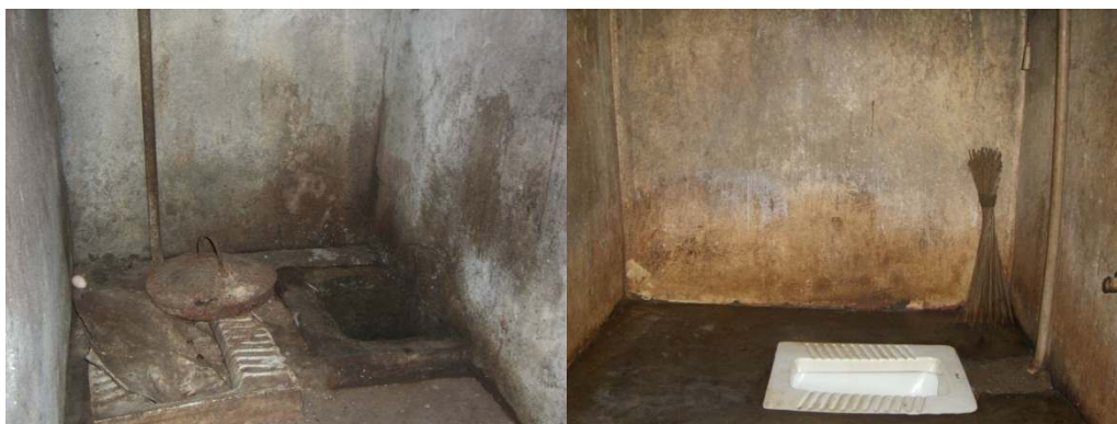
Photograph 5: Old dilapidated, colonial toilet facility for female inmates at PA (Left) and the semi modern toilet at PB (Right) (FP)
