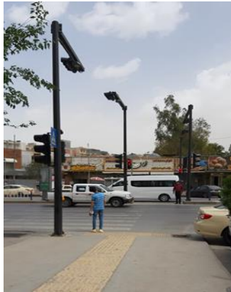
Figure 20: Adding traffic lights on point in Salim Street (Ref: the Researcher)
