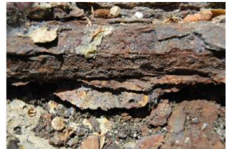
(g) Rebar so corroded that has a thick oxide layer in the surface
