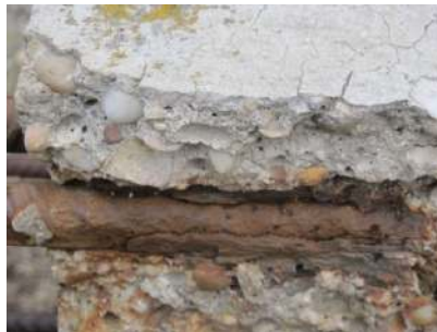
(f) Old rust sjhowng parallel-to-the-bar layering
