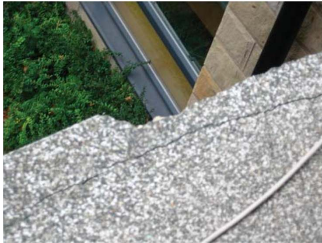
Figure 5: Concrete degradation creating an Health & Safety issue.
