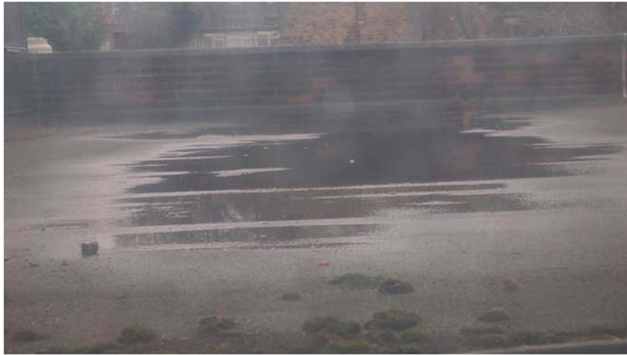
Figure 7: Ponding and moss growth to flat roof areas.
