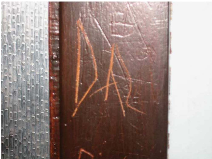
Figure 8: User damage (Graffiti).
