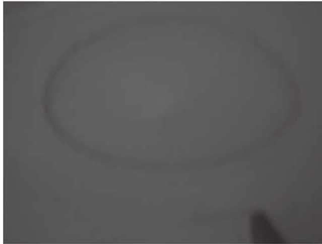
Figure 9: Damage to ceiling caused by service failure.
