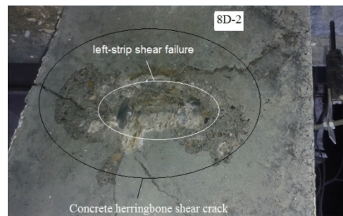
(g) Concrete herringbone shear crack
