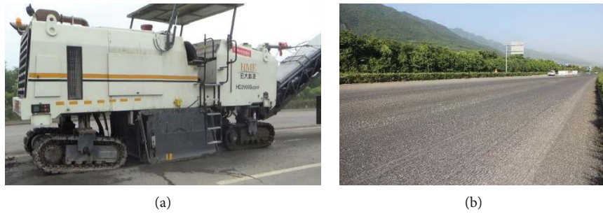
FIGURE 7: Milling operation on test field: (a) milling machine in the field and (b) milling surface in the field.
