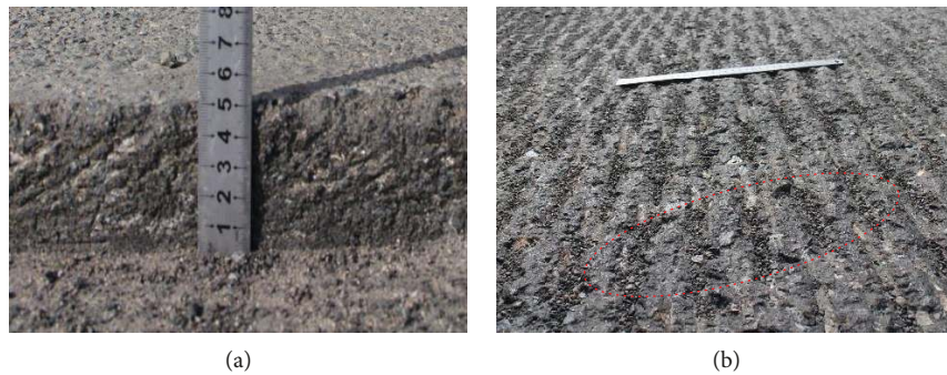
FIGURE 8: Milled pavement surface in the field: (a) milling depth after operation and (b) milling texture in the field.
